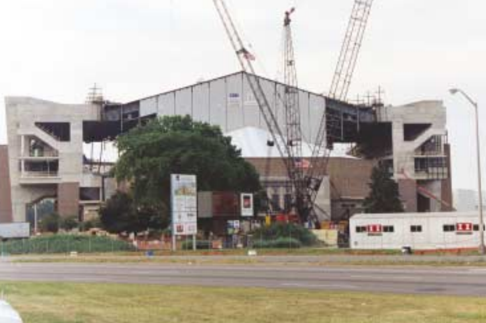
View of coliseum at the new raised height of 41'-10" above the previous position. The final elevation of the peak is roughly 120' above grade.
