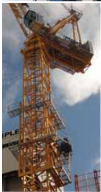
Potain tower cranes from D&G Hoist and Crane Hire's fleet at work in the city of Perth, Australia
