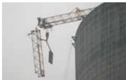
After removal of the bottom jib connection bolts, the fold-down jib section is trolleyed inwards over the cooling tower and lowered to the ground
