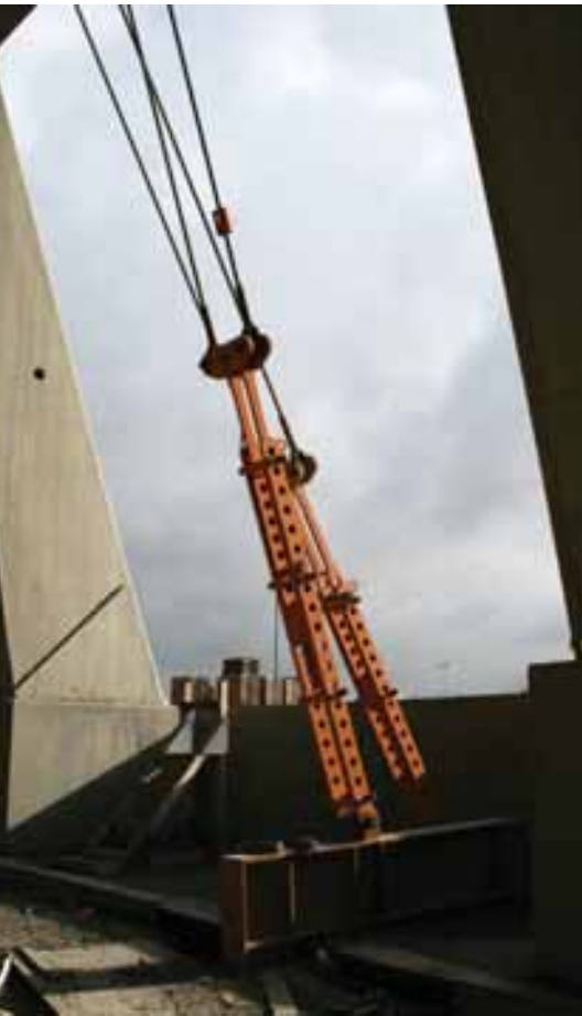
Guy anchorage of the Liebherr 280 EC-H
