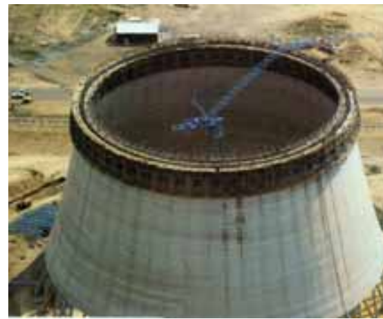
A 165 m high cooling tower with 104 m diameter built for the Lethabo power station in South Africa with the help of an Elba Kaiser HBK160 articulated jib tower crane
