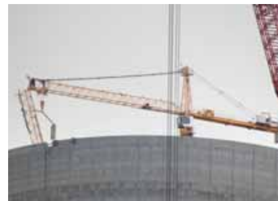
The last jib section being dismantled before the crane can climb down inside the cooling tower
