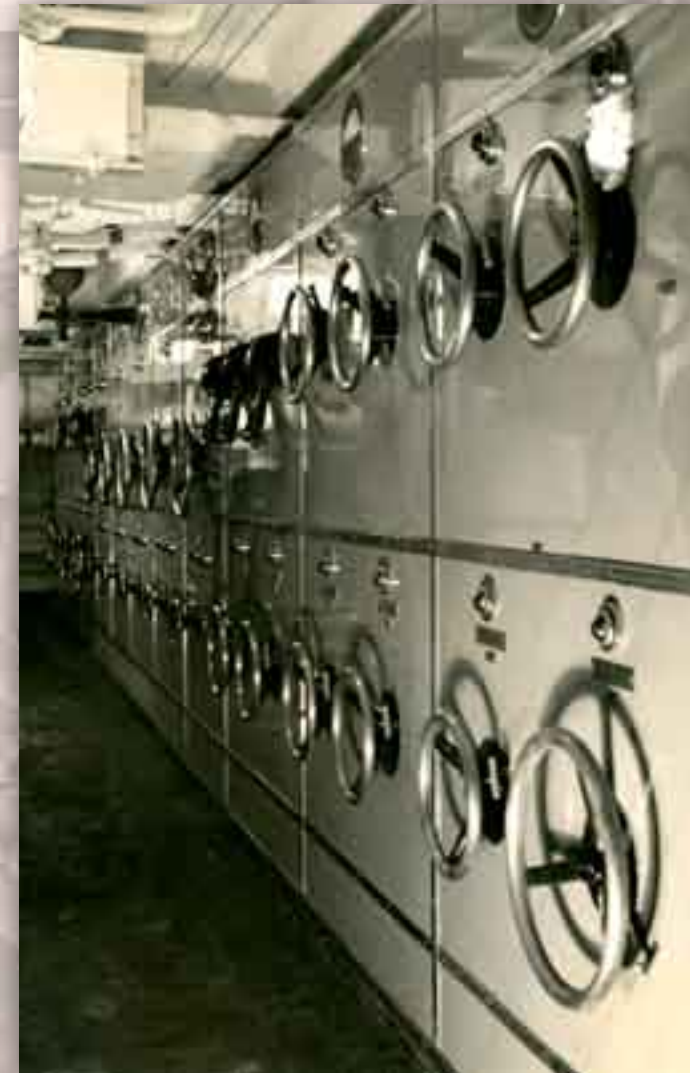
The main switch panel of the 'ss Nieuw Amsterdam' in 1936.
