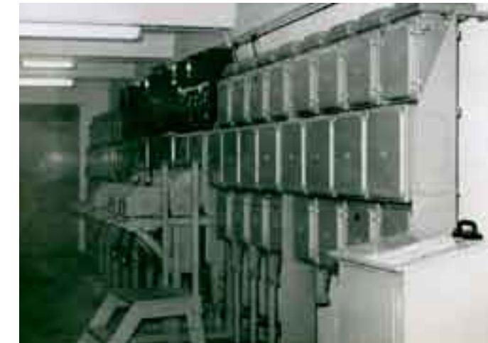
The workshop with switch boxes.
