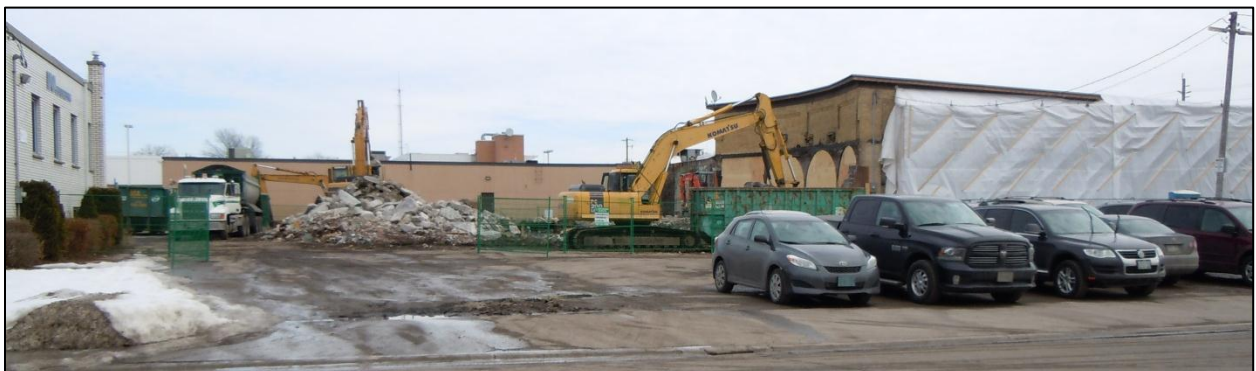
Figure 2 – East facing view of subject lands, from Waterloo Street with rear addition being demolished and removed.
