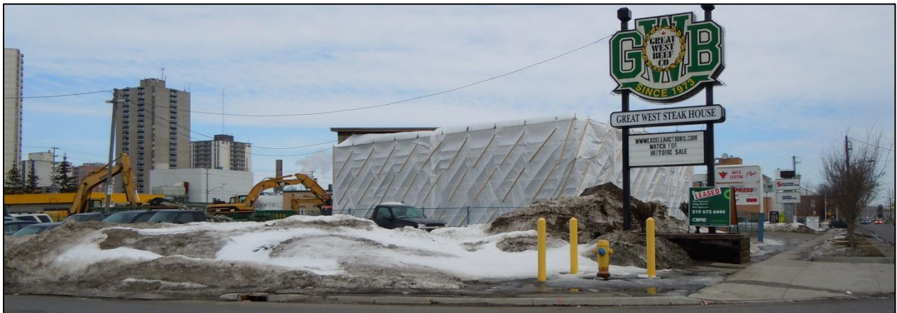
Figure 1 – East facing view of subject lands, known as 240 Waterloo Street from intersection of Waterloo & Horton.
