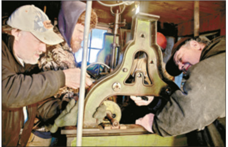
Courthouse clock is removed from bell tower to be transported to restoration shop.
