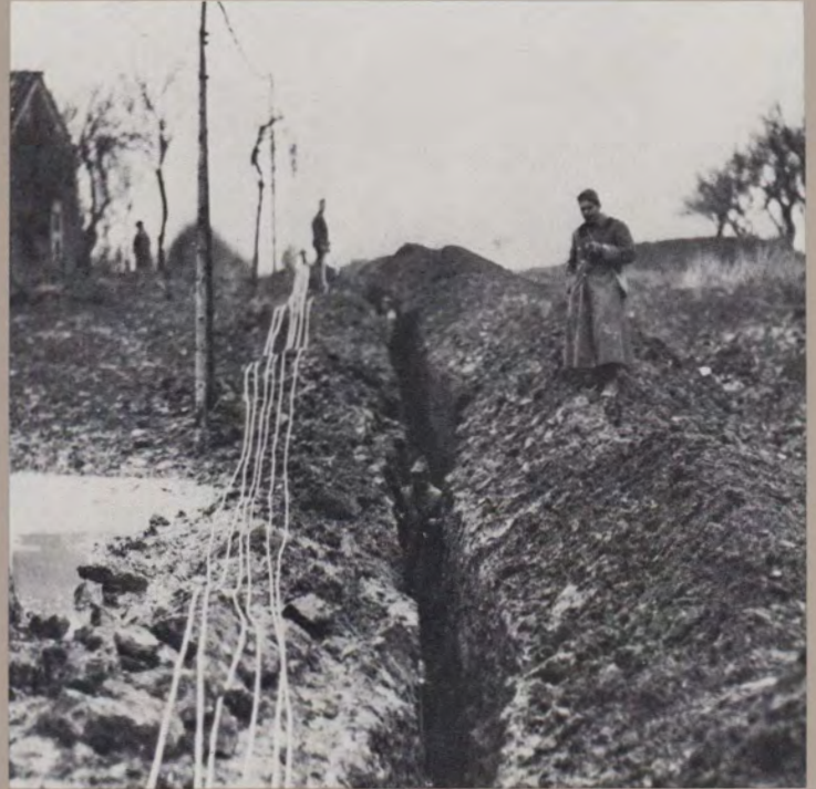
Trenches and World War I go together. This one near Ausauville, France, was for telephone cable. Like many during the war it was dug under continuous German battery gun fire. The date on this is 1918.
