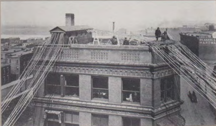
This was the telephone exchange in Kansas City, Mo. in 1895, when WE installers were putting in a new exchange. All wires still came in over the rooftops.
