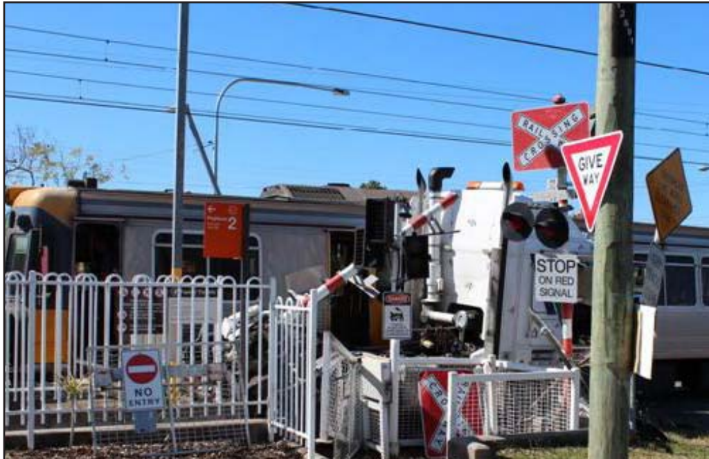
Figure 6: Damage to rail infrastructure
