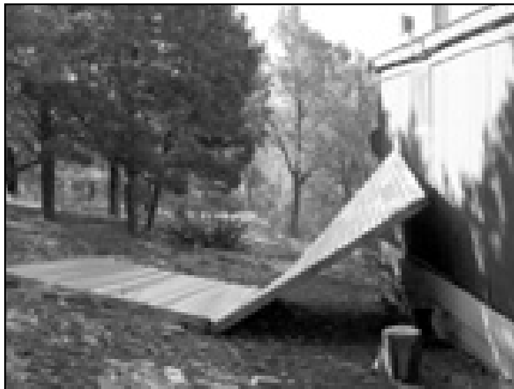
High winds took Barbara Jordan's porch roof off and threw it over the house.
