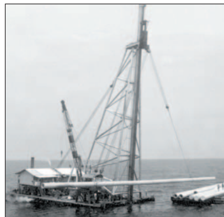
Pile driving barge Rotterdam handling a 36in prestressed concrete pile in Lake Maracaibo in the 1950s.
