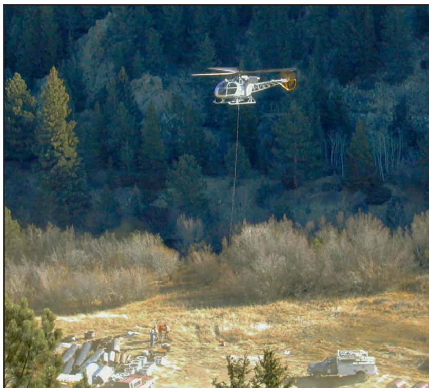
A helicopter transported steel pipe during the repair of the Barker Gravity Line. Photo courtesy City of Boulder
