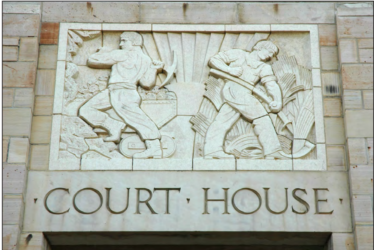
Boulder County's economy was founded on mining and agriculture, as depicted in this ArtDeco bas relief sculpture over the front entrance of the present-day Boulder County Courthouse. Pettem photo
