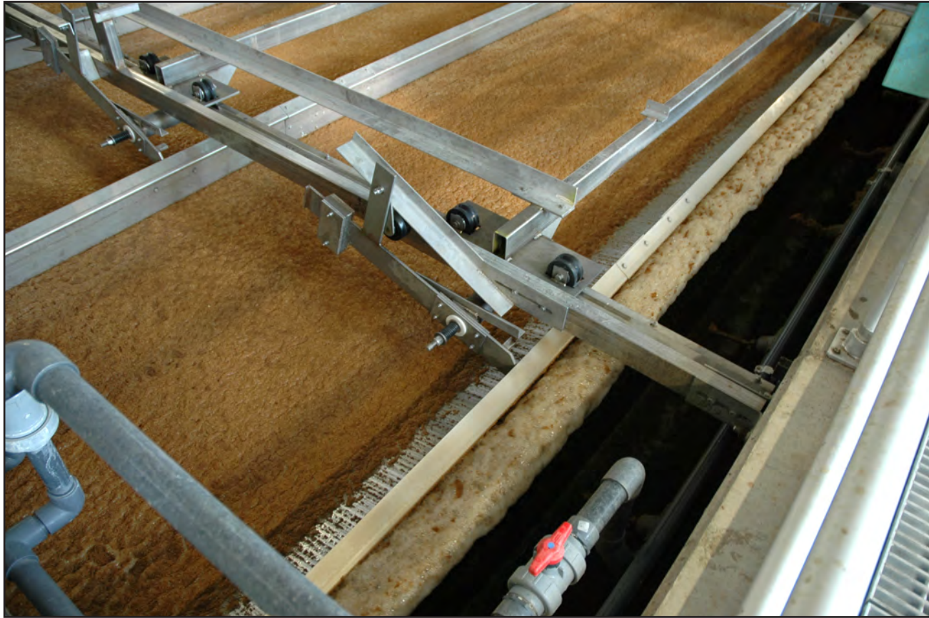
At the Boulder Reservoir Water Treatment Plant, residuals are scraped off of the water's surface. Pettem photo, 2013.
