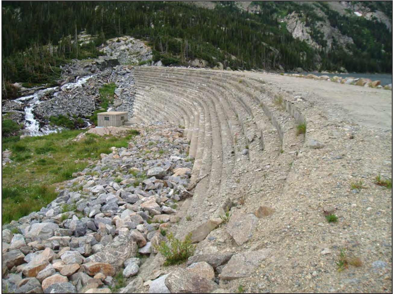
In 1989, roller-compacted concrete was installed on the downstream face of Goose Lake. Photo courtesy City of Boulder
