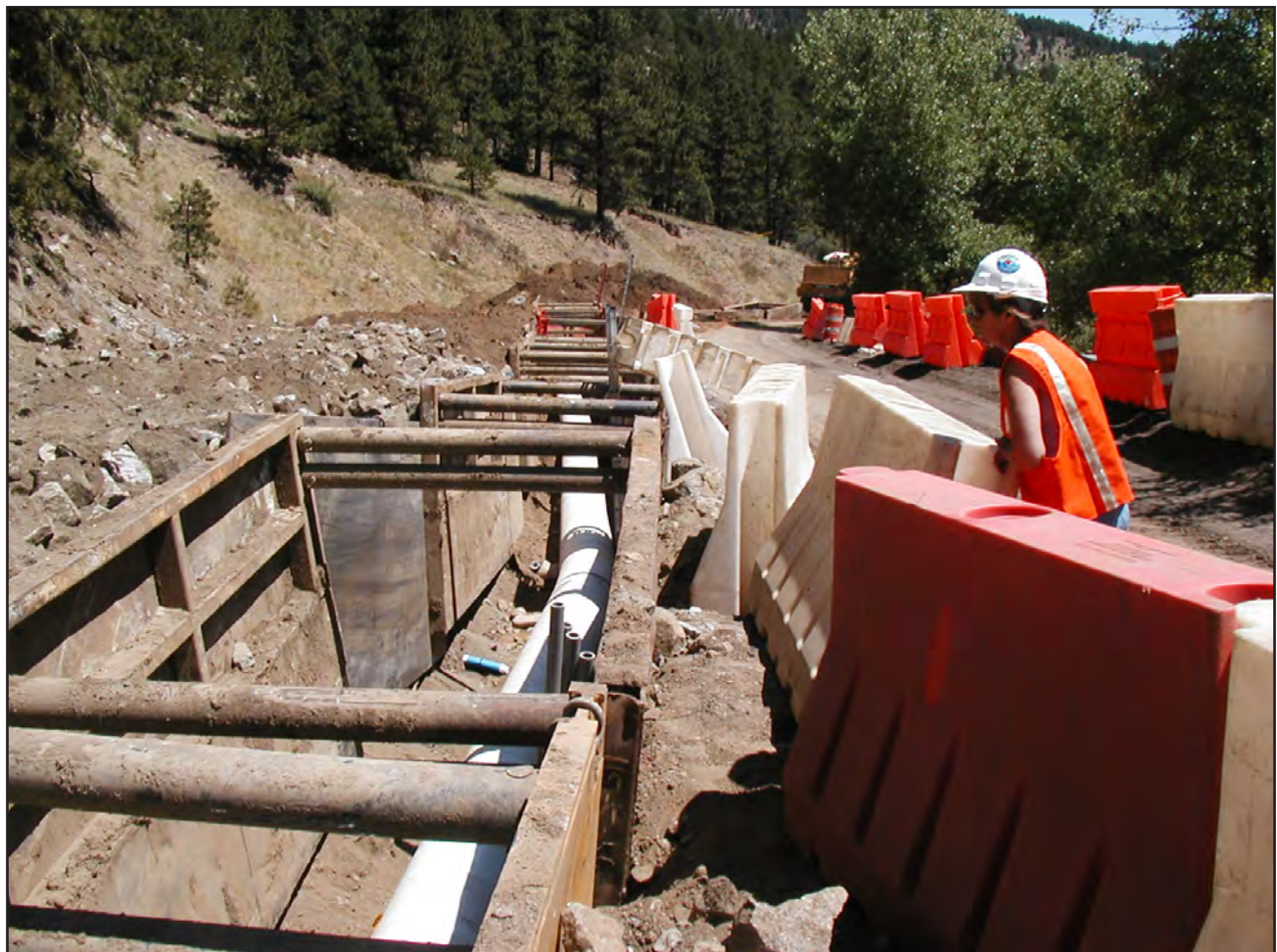
After the City was required to relocate the Lakewood Pipeline into Sugarloaf Road, its reconstruction disrupted the lives of Sugarloaf Mountain residents. The road was (and still is) their only direct access to Boulder. Photo courtesy City of Boulder
