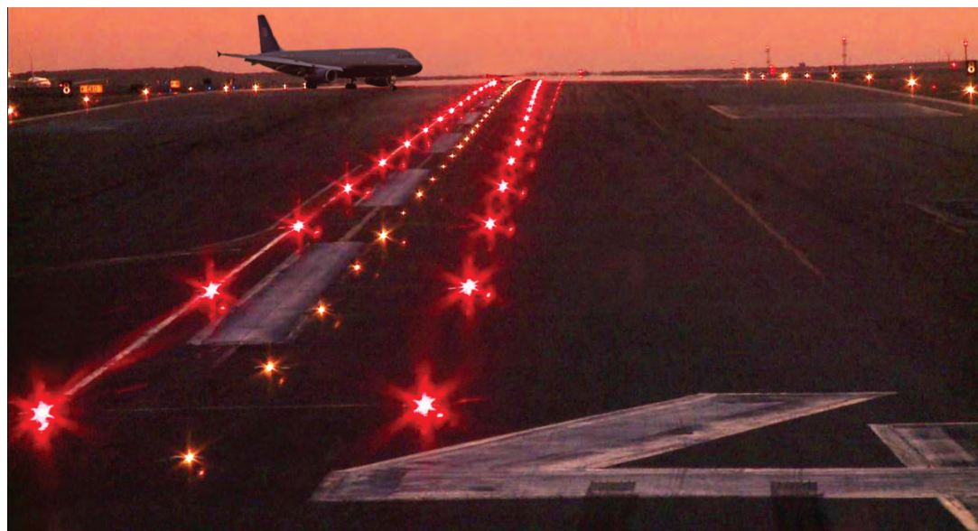
Figure 33–4 A view of the in-pavement Runway Status Lights at the Los Angeles International Airport.
