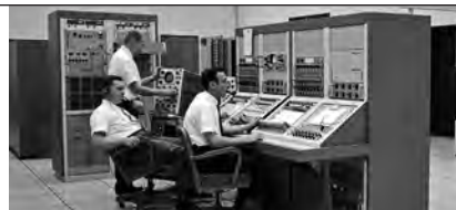
LASA maintenance console
