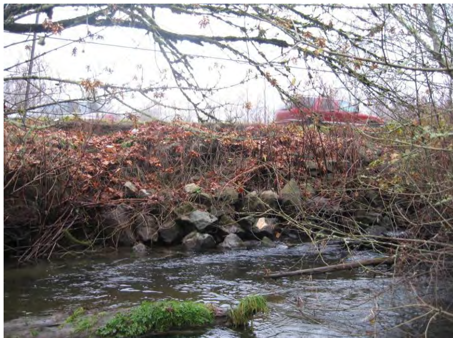
Figure 6. Union River, downstream from bridge, eroding highway embankment.
