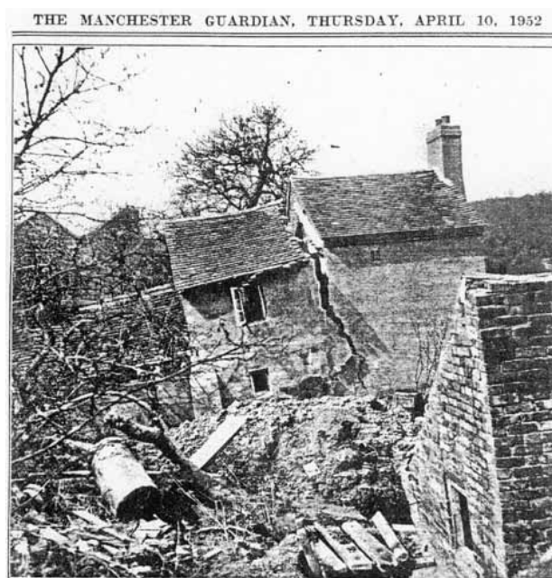
Figure 12 Pear Tree Cottage, damaged by the 1952 Jackfield landslide and demolished the following year (Manchester Guardian, 10 th April 1952).
