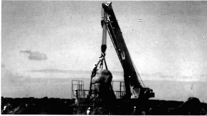
Reconstruction of Ahu Tongariki underway in 1993 using the crane donated by Tadano Corporation (photo by R. Morales).
