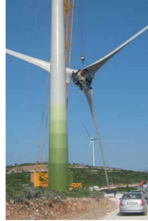
Location with excellent wind conditions: Kedros wind farm with six ENERCON E-82/2.3 MW.
