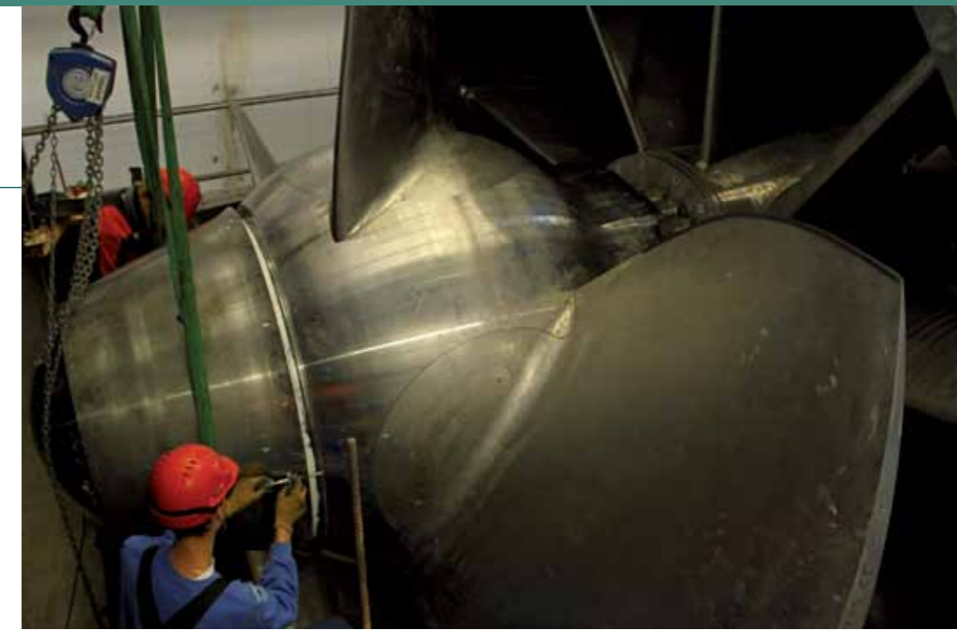
Second turbine on the grid: After completing several weeks of testing, ENERCON successfully started normal operation at the Weser hydropower plant.
