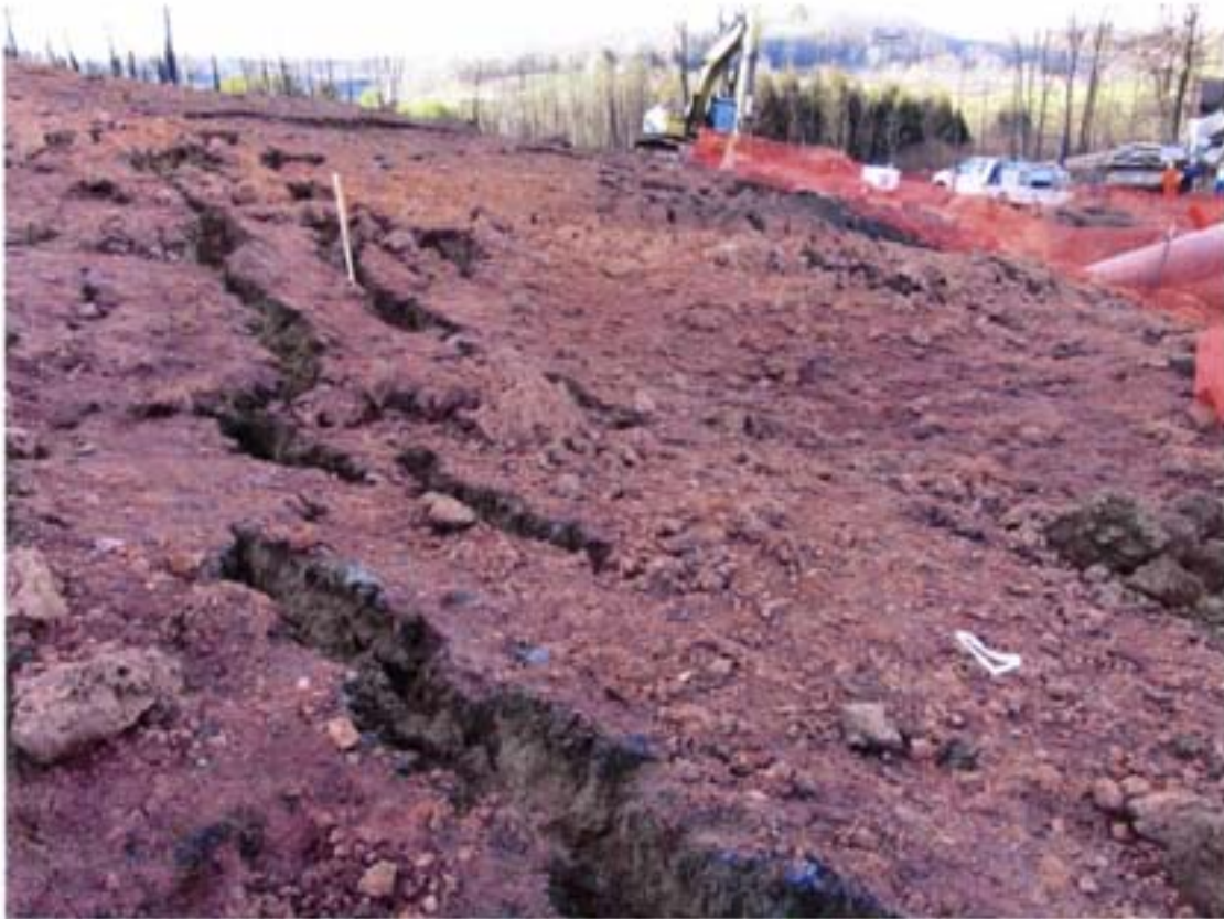
Figure 3. Photograph of Hillside Post-Failure and located above Pipeline Failure
