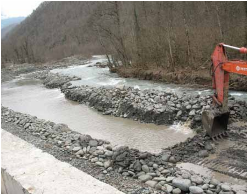
The pollution of Mzymta river and its tributaries was caused by barbaric construction methods
