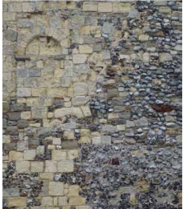
Signs of earthquake damage? The rebuilt walls of St Mary's Church Rory Walsh © RGS-IBG Discovering Britain
