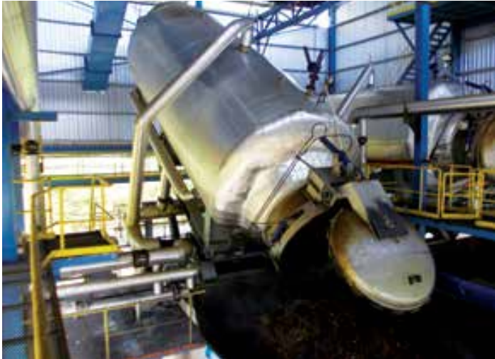
The new tilting steriliser installed in Segaria Palm Oil Mill in Sabah
