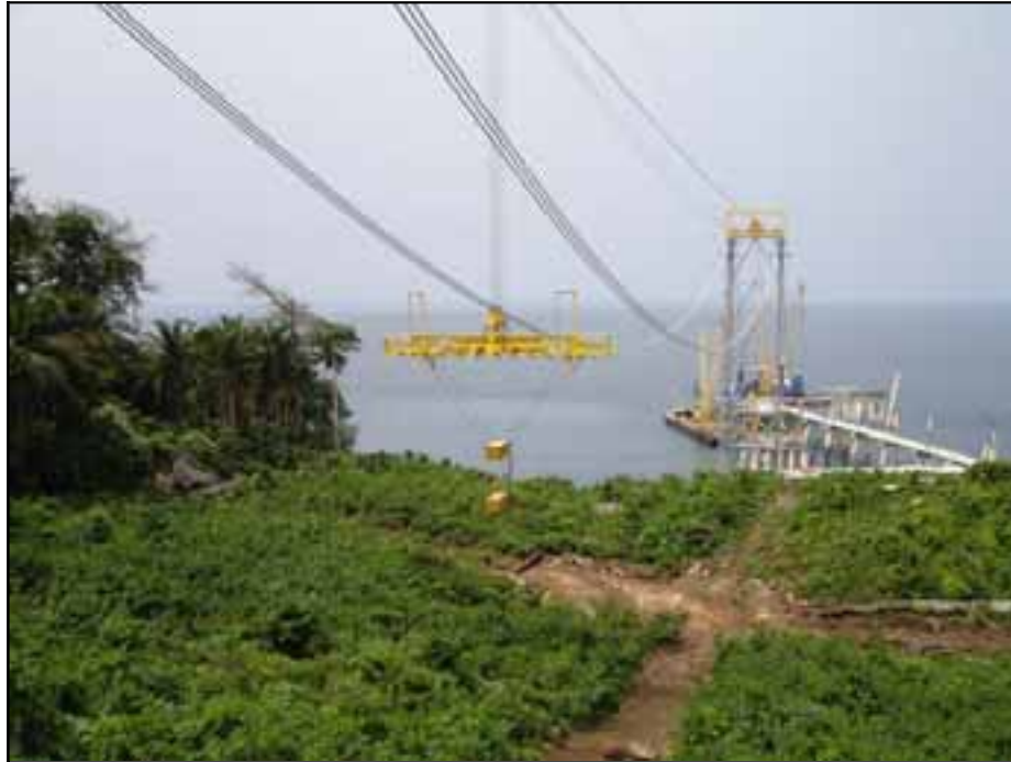
Test Run of Work Platform Used to Install Cable Clamps and Suspender Wires
