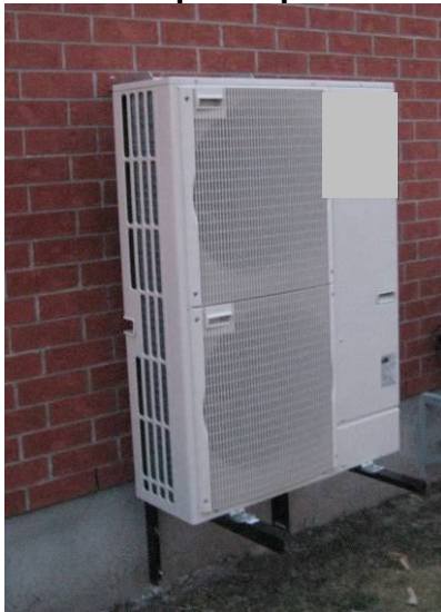
Ducted cold climate air source heat pump
