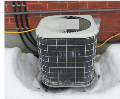
Central A/C + furnace
