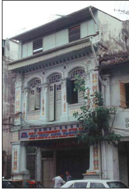
PLATE 3. Deteriorated Shophouses in Niucheshui
