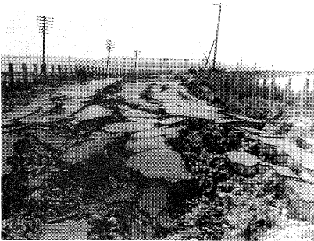
Figure 4: Photograph showing severe lateral spreading of embankment of road across Napier Harbour. (Courtesy of the Alexander Turnbull Library, Tyndall Collection, Wellington).
