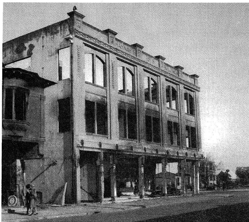
Figure 11: (a) A successful reinforced concrete building. Hannah's shoe shop, Napier, a "corner building", MRF + concrete block infill. (Courtesy of the Alexander Turnbull Library, Wellington).
