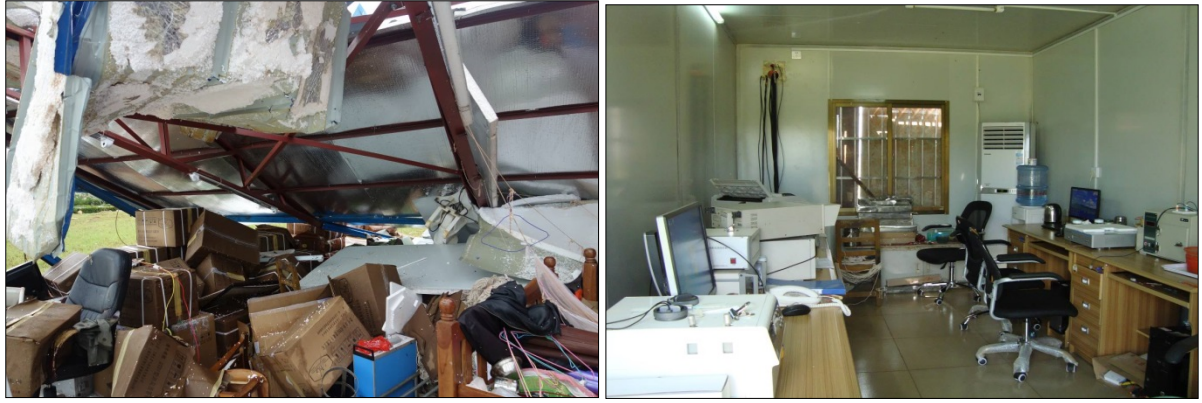
Fig. 2.4 left) On July 18, 2014, due to the Super Typhoon Rammasun, the temporary duty rooms at Haikou upper-air observatory, Haikou Meteorological Bureau, collapsed. Computers, printers, radiosonde and other equipment in the rooms were all damaged. Right) On July 19, 2014, Haikou Meteorological Bureau equipped computers, printers, etc. for Haikou upper-air observatory.
