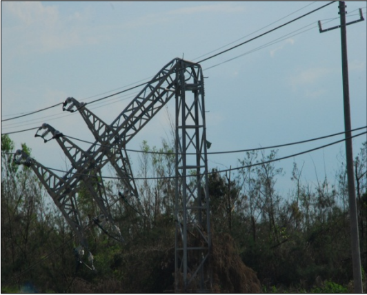
Fig 1.8e Damages by RAMMASUN in Hainan
