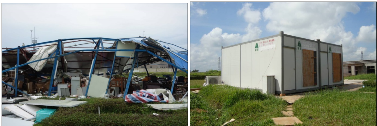
Fig. 2.3 left) On July 18, 2014, due to the Super Typhoon Rammasun, the temporary duty rooms at Haikou upper-air observatory, Haikou Meteorological Bureau, collapsed. Right) On July 23, 2014, Haikou Meteorological Bureau rebuilt the rooms.
