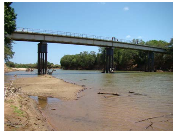
The Bu'aale bridge in March 2008. This bridge has very high clearance and SWALIM maintains a river gauge below
