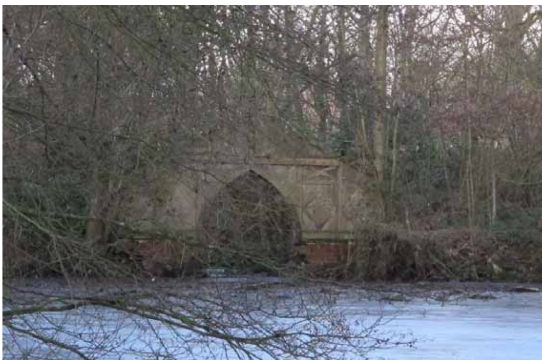
Figure 12: Clear vegetation round the ruins of the boathouse and stabilise the structure to prevent further deterioration
