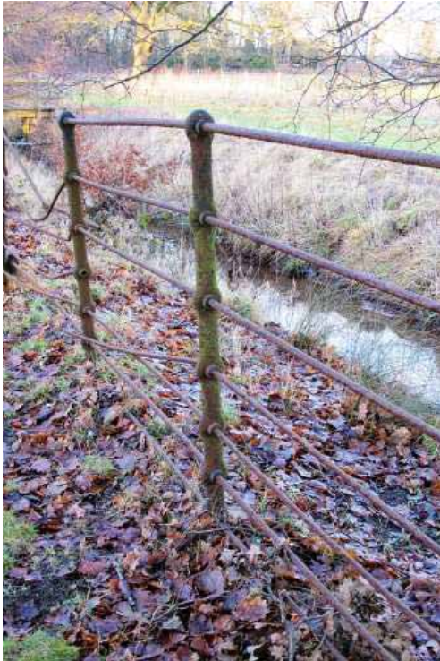
Figure 25: The railing at the end of the East Prospect will be repaired
