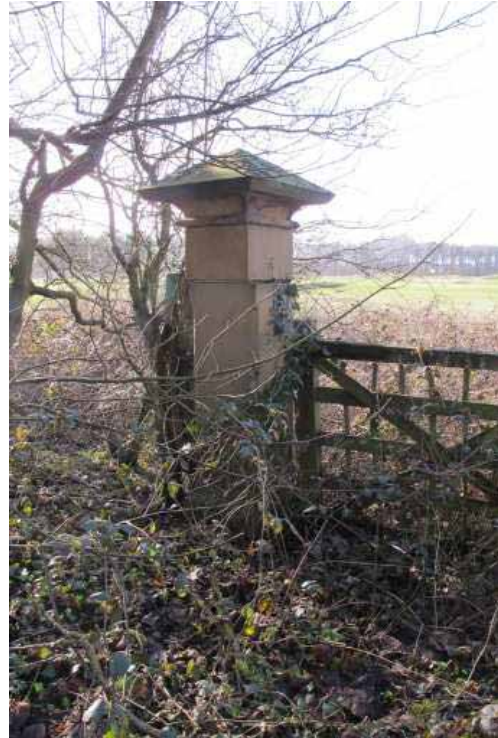
Figure 26: The gateway on the former drive to Hey House Lodge will be restored as a viewing point across the golf course
