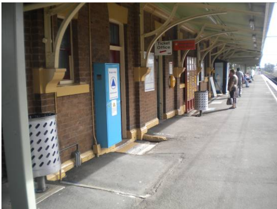
Uneven surface on Platform 1
