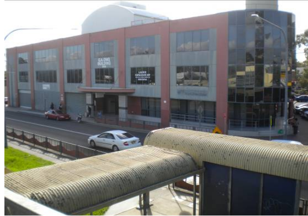
Deteriorated bus shelter awnings viewed from ramp
