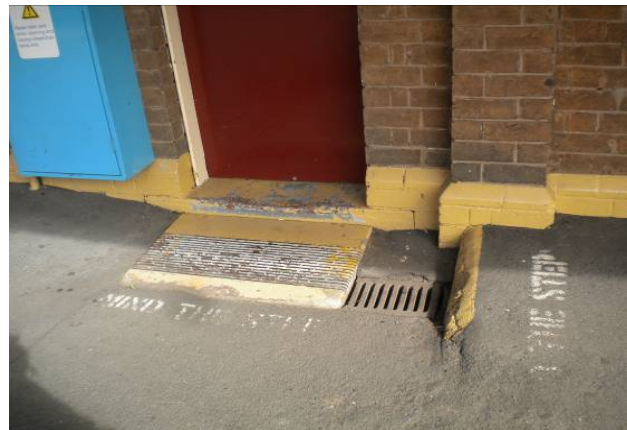
Drainage and uneven platform levels
