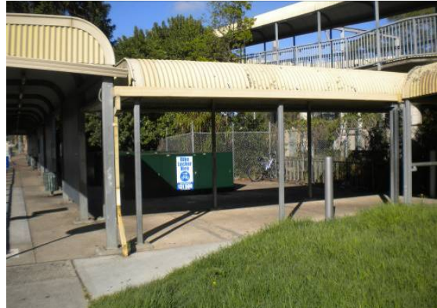
Close up of station entrance in Ingleburn Road indicating deteriorated bus canopies
