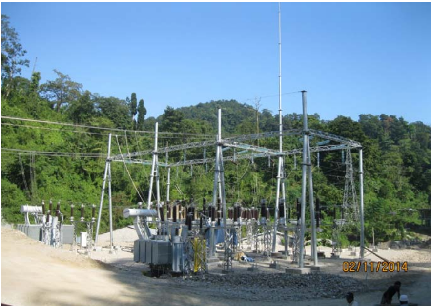
Figure 15: Substation at powerhouse
