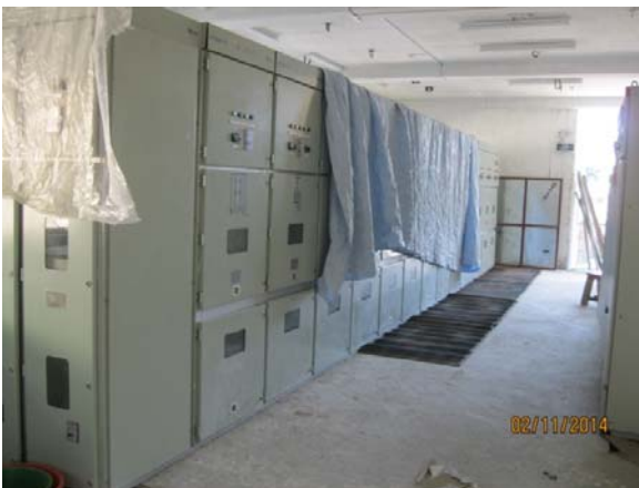
Control Panel PH
