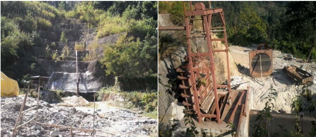
Figure 6: Air vent pipe installation at inlet portal and repairing of valve gate
