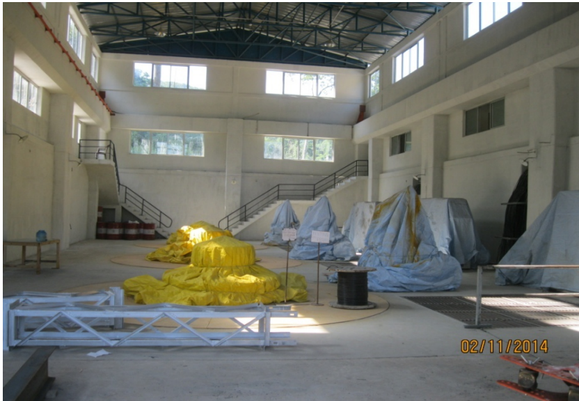
Figure 11: Electro Mechanical installation
