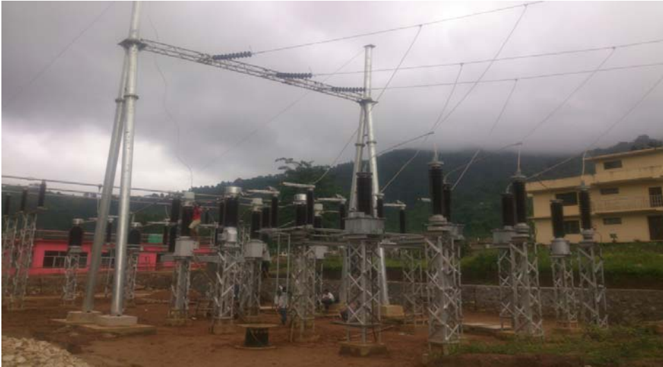
Figure 14: Substation at Godak
