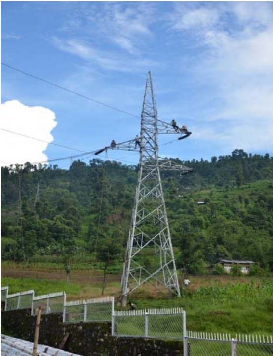
Figure 13 T#36, Type DD near Substation at Godak
