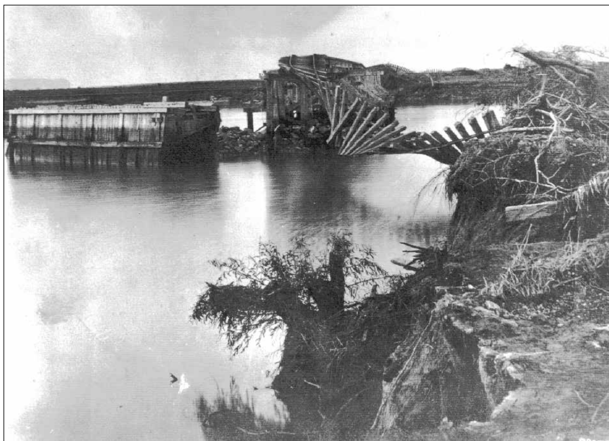
Figure 1.7: Damage caused to road and rail bridges by flooding of the Ngaruroro River at Waitangi in 1897. (photo: Alexander Turnbull Library 61690 ½ - print donated by C. Athol Williams).
