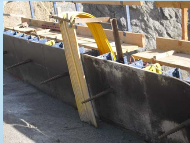
CVC against Formwork and RCC poured at same time
