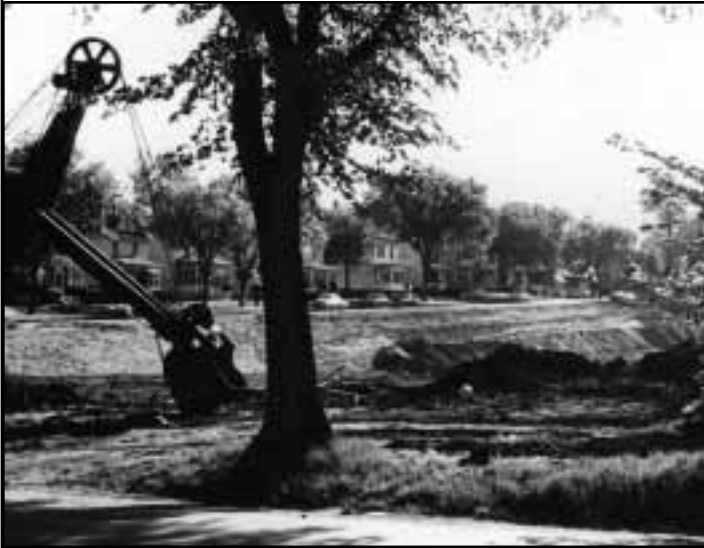
Interstate 94 construction, looking toward St. Anthony and St. Albans, 1966. (Courtesy of the Minnesota Historical Society, location no. HE3.81 r75. Reprinted with permission.)
