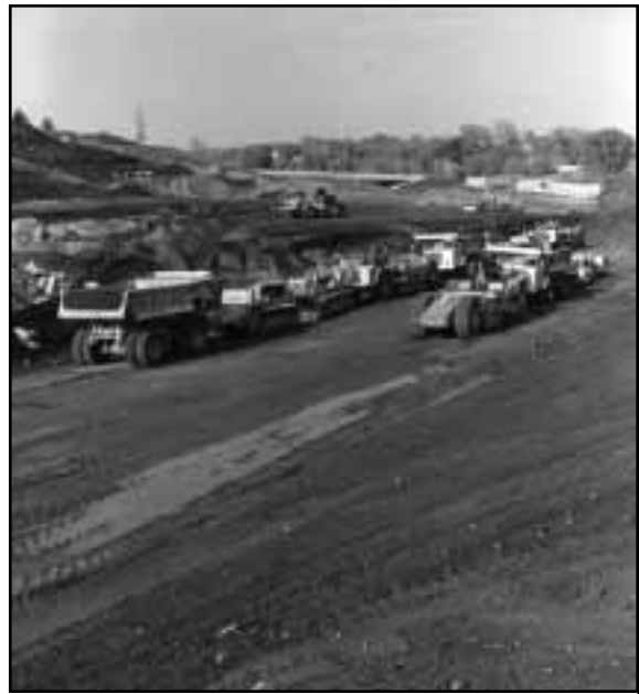
I-35E construction, St. Paul, 1971. (Photo by Henry Benbrooke Hall, courtesy of the Minnesota Historical Society, location no. Collection III.44.109, negative no. 014266-8. Reprinted with permission.)
