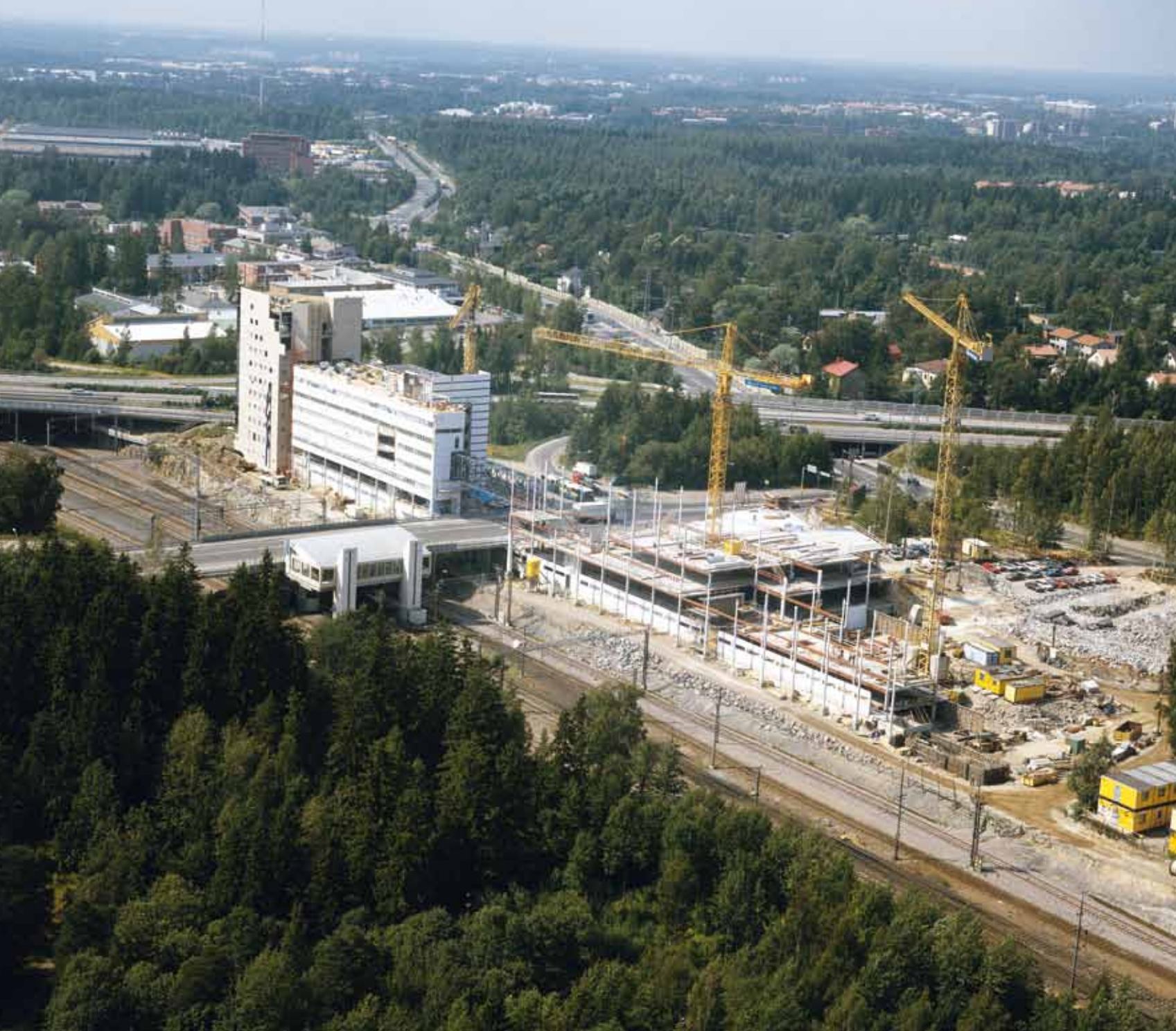
YIT's new head office under construction in Helsinki in 1991, during the economic recession.
