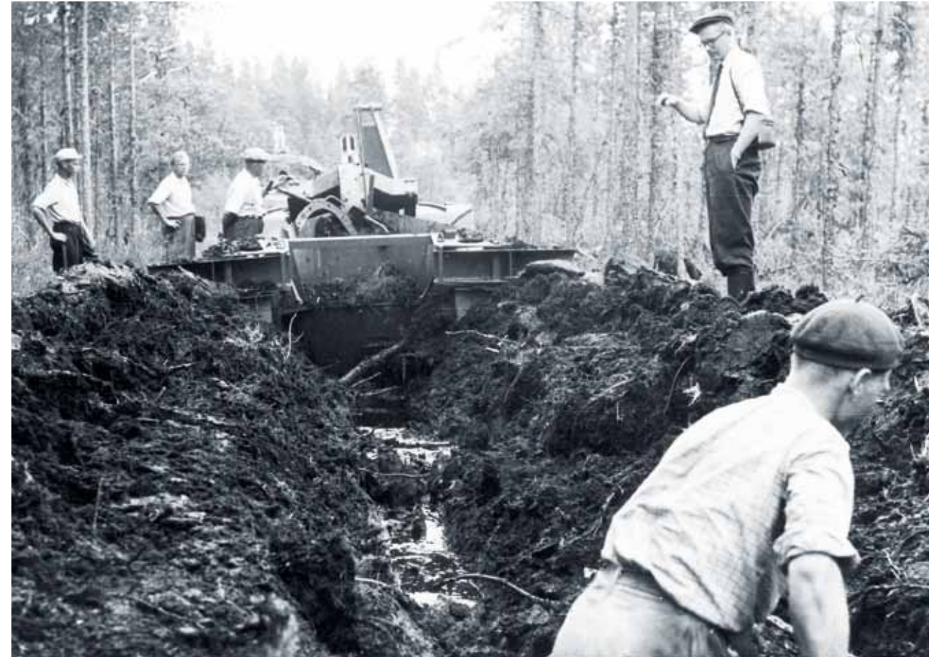
Bogs were encroaching on woodlands. Drainage was required to turn these areas into productive forests. In the 1950s, the Pellonraivaus company developed a tractor-pulled plough that was an excellent tool for this purpose.
