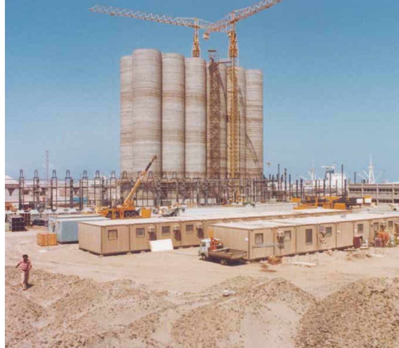
Vesto Oy built a grain silo and bagging plant in Hodeidah, Yemen, on the shores of the Red Sea in 1978–1979.
