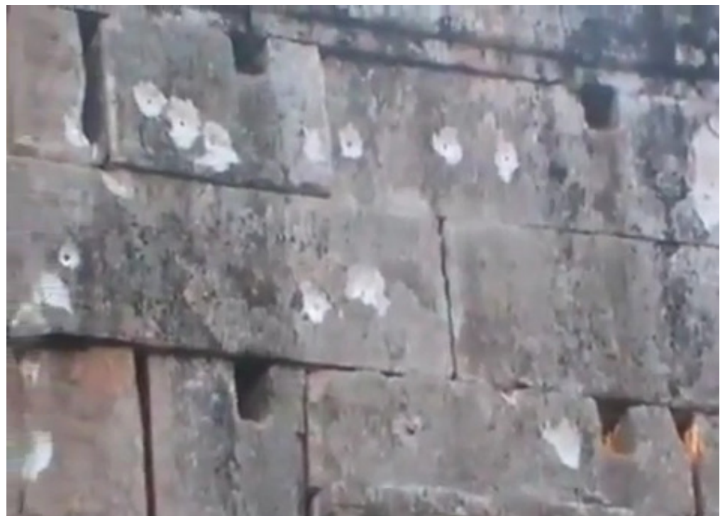
Figure 9: Shelling damage at Deir Sunbel 121
