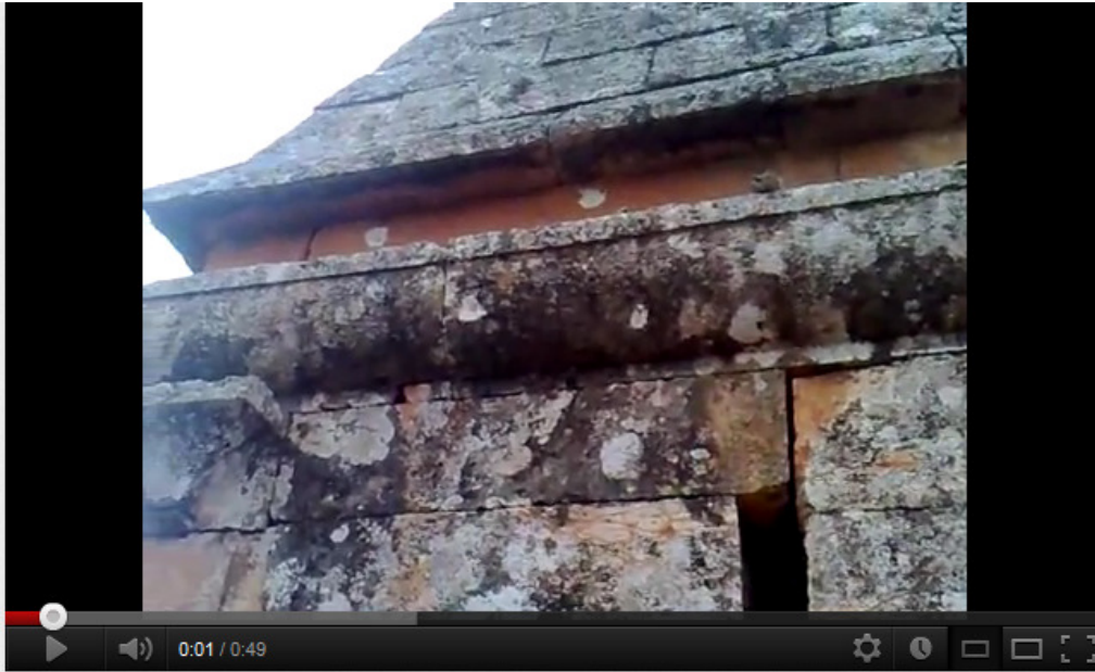
Figure 10 Shelling / gunfire damage to tomb at al-Bara 122
