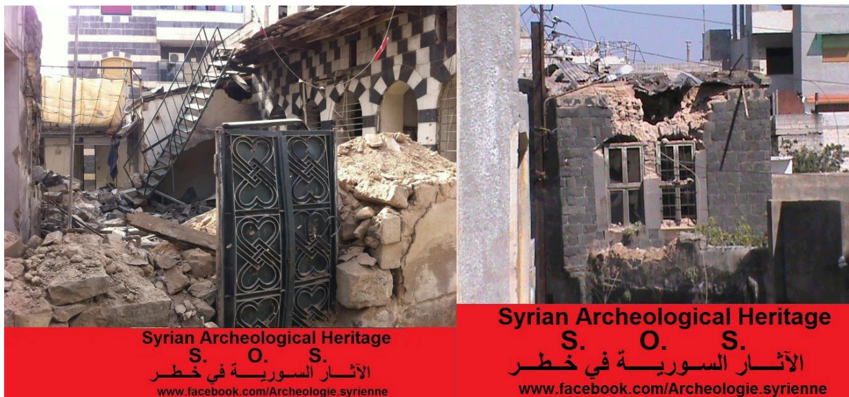
Figure 26: Damage to ancient houses in Homs 202
