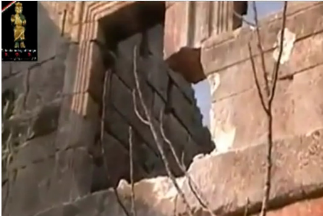
Figure 8: Shelling damage at Deir Sunbel 120
