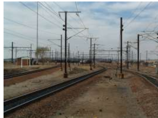
Pyramid yard, transfer point from AC to DC voltage railway lines. (7.13)
