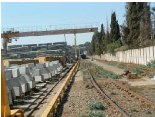
Concrete sleeper plant in Vulkania Industrial area, Brakpan. (4.1.32)
