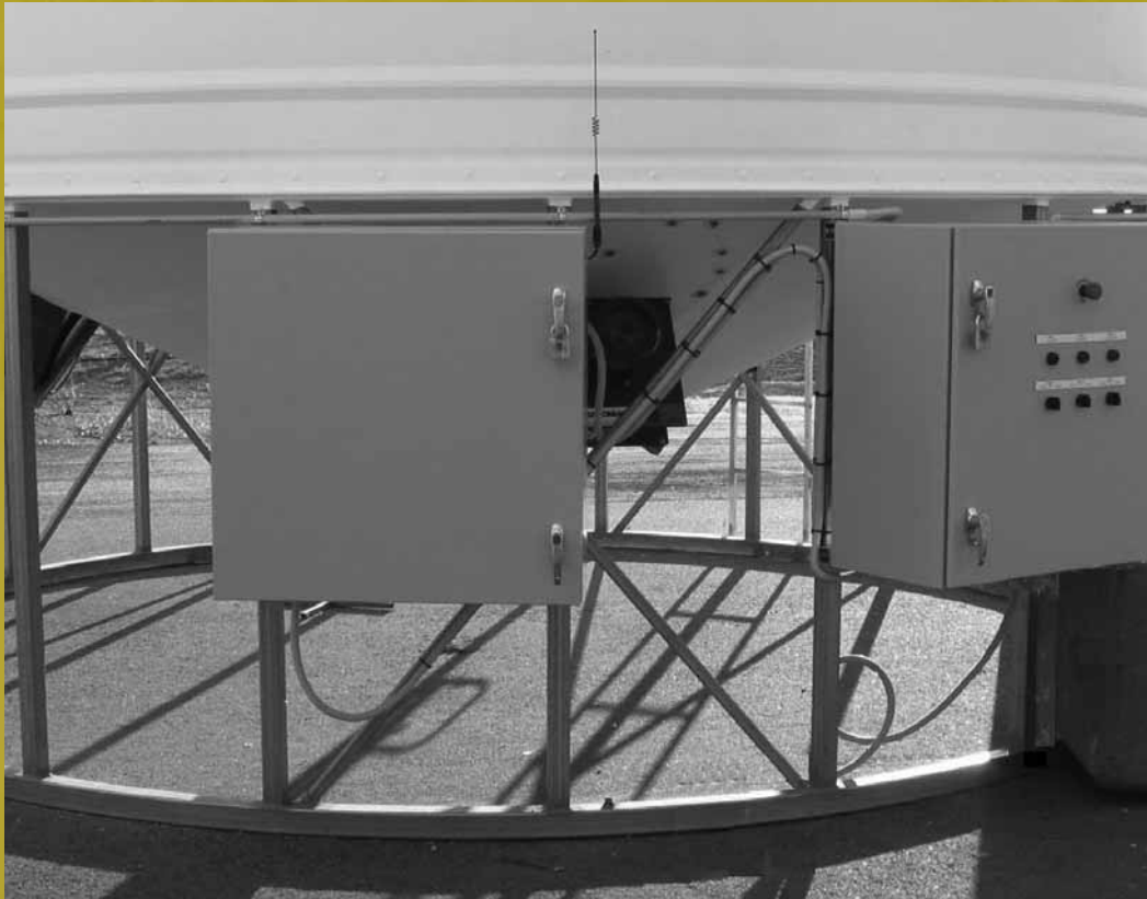
The new Adaptive Discounting Controller can control three aeration functions at once: cooling, drying and maintenance.
