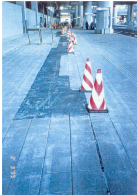
Figure 4. Cracked area of walkway (Kaiyo Kogyo, 1995)
