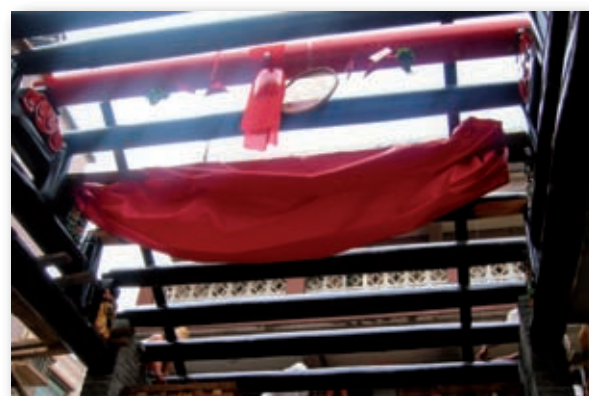
Raising the principal beam, Lam Ancestral Hall, Hang Ha Po, Lam Tsuen (Provided by Lam Ancestral Hall)
