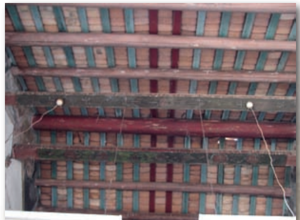
Roof of main hall, Chan Ancestral Hall, She Shan Village (Photography by Lo Wai Ling)
