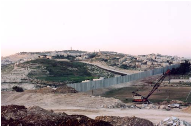
Construction of the concrete wall in Abu Dis, East Jerusalem, March 2004. © AI
