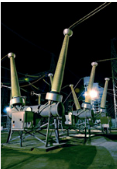
THE GCCIA PROJECT IN THE GULF INTERCONNECTS THE POWER GRIDS OF ITS SIX MEMBER COUNTRIES.
