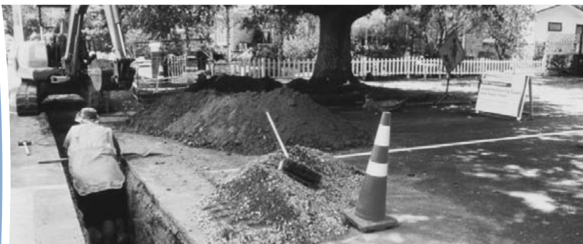
Water supply pipes on Norton Road being replaced with new long-lasting PVC pipes.
