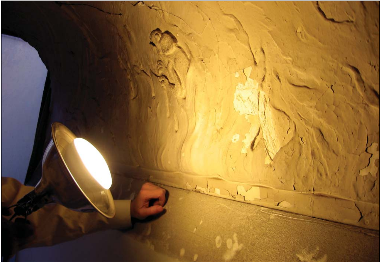
Figure 4.6. Curved cornice on East wall, with removed appliqué portion (WHIT2010.P2), November 2009. Old World chameleon figure is further evidence of applied pre-cast element, surrounded by a series of applied flames to visually and physically fix the element in place (L. Drapala, 2009).
