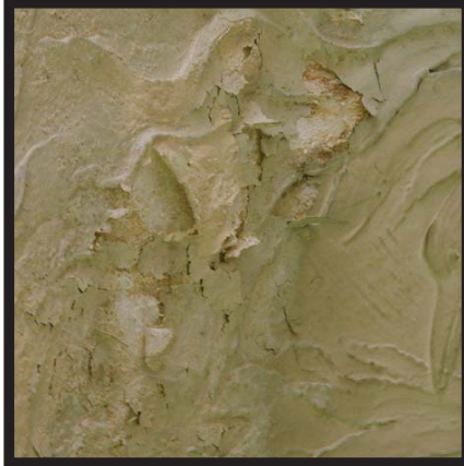
(b) vulnerable plaster due to paint loss
