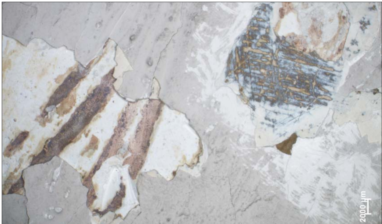
Figure 7.6. Paint exposure on fallen cornice panel, revealing mauve color in creasing, 7.1x mag, reflected light (L.Drapala, 2010).
