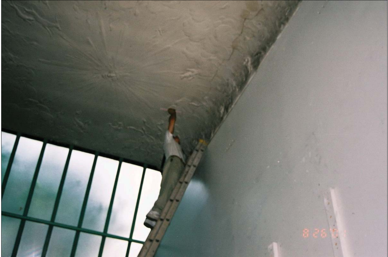
Figure 1.12. Brice Bowman (SuperStructures) measuring cracks in plaster, 2001 (Archives of the New York Studio School).
