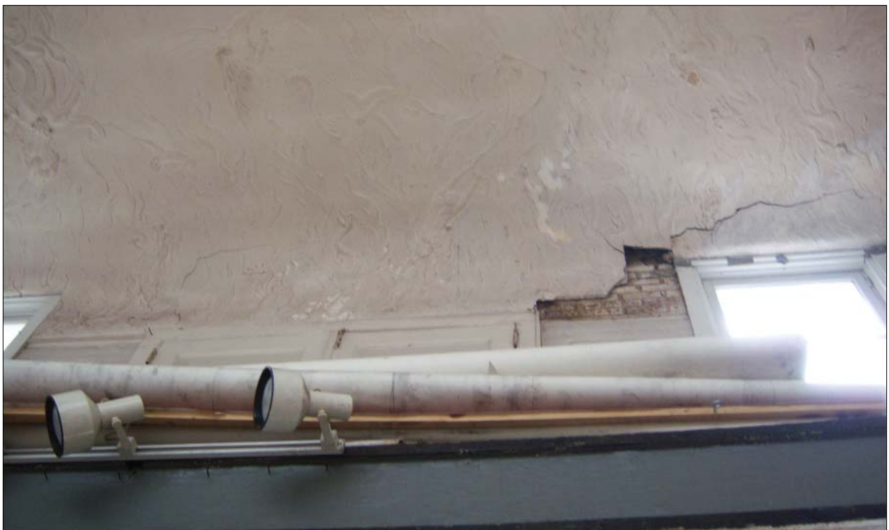
Figure 1.13. Following the cornice failure (L. Drapala, 2009).
