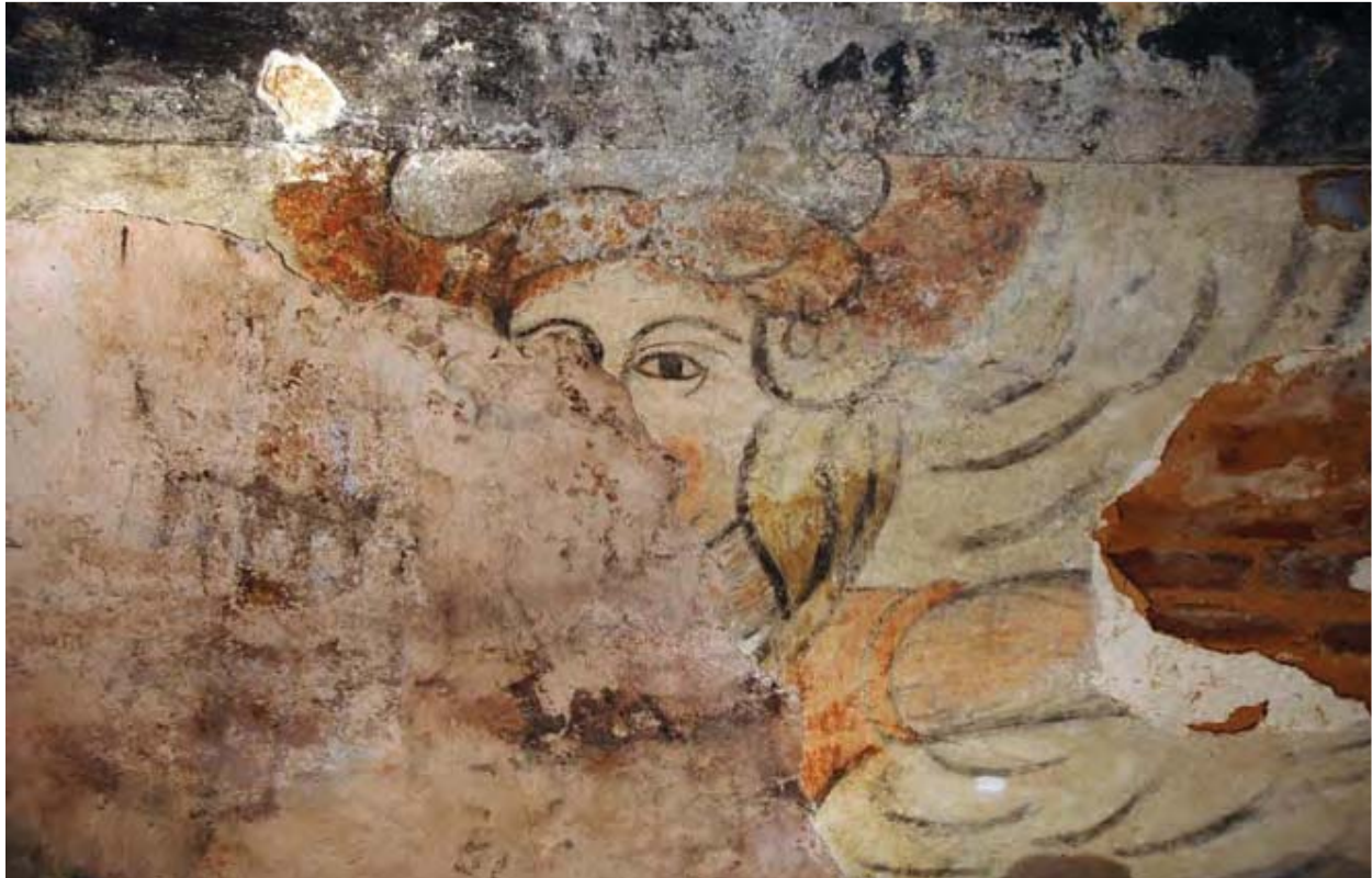
Figure 1.2. Detail of exposed Southwest pendentive at the Rosario Chapel, Iglesia San Jose in Puerto Rico. (K. Johnston, 2008)
