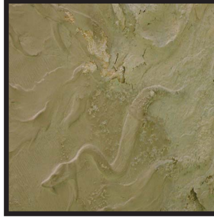
(c) loss due to extensive pitting
