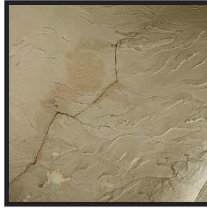
(c) staining due to prior treatment
