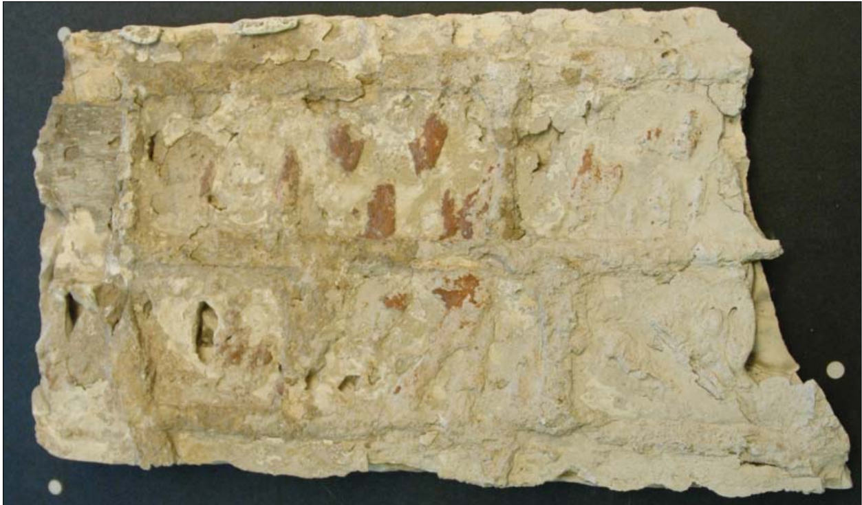
Figure 4.3. Back of P1, cornice segment that had fallen in May, 2008. Evidence of keying to the masonry is visible in the mortar joint imprint (L. Drapala, 2009).
