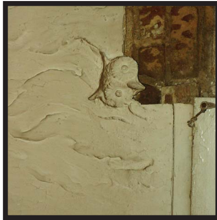
(a) cornice failure
