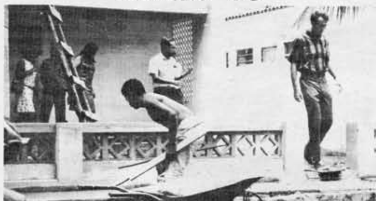
KENT GOODYEAR leads the group out of one of the newly finished parts of a housing construction project, which is designed for the poor families of the region.
