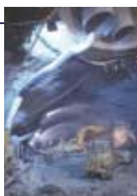
Excavating the underground cavern that will house the ATLAS experiment at the LHC
