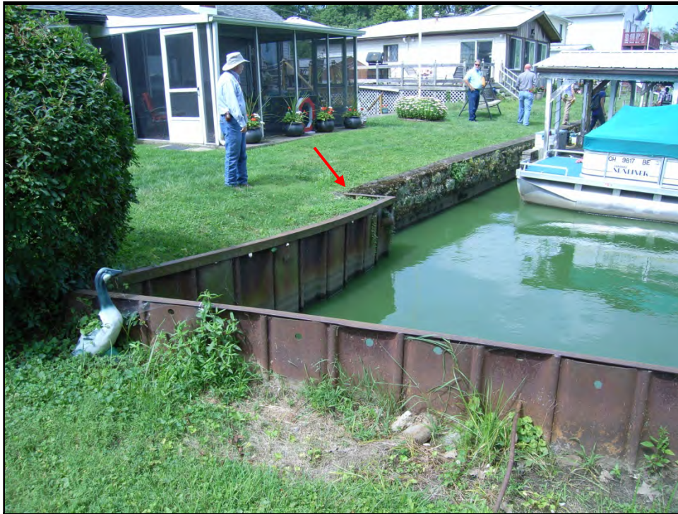
BUCKEYE LAKE 25 AUGUST 2014 Photo 001 – Beginning of west embankment masonry wall as seen from the west abutment.
