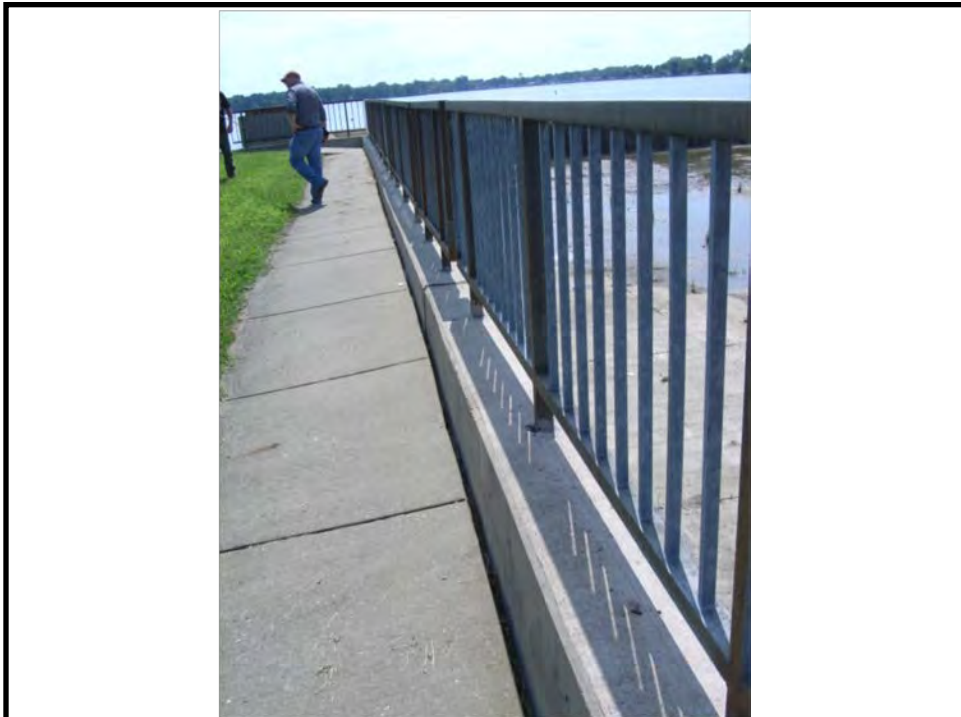
BUCKEYE LAKE 25 AUGUST 2014 Photo 022 – Settlement along sidewalk behind eastern training wall at Sellers Point spillway.
