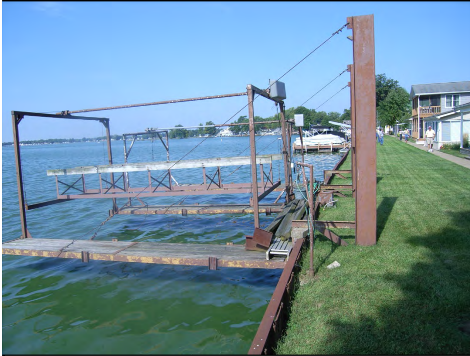
BUCKEYE LAKE 25 AUGUST 2014 Photo 035 – Dock structures cantilevering off of the dam put stress on the sheet piling that it was not designed for.
