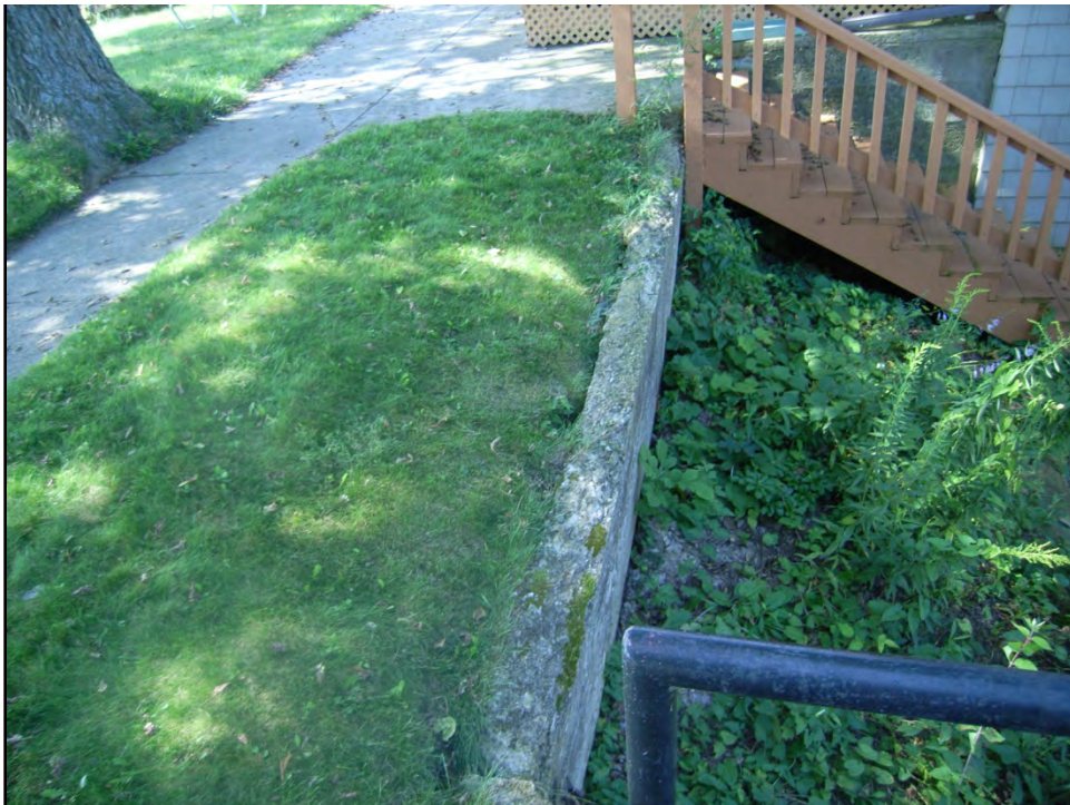
BUCKEYE LAKE 25 AUGUST 2014 Photo 038 – Failing shallow retaining wall.
