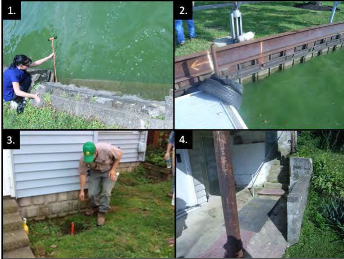
Figure 3. Other Wall and Seepage Observations 1) Displaced portion of masonry wall 2) Numerous rust holes observed in sheetpiling 3) Several depressions possibly due to boils, together with very shallow ground water conditions, were observed 4) Location of persistent seepage near Black Diamond Point
