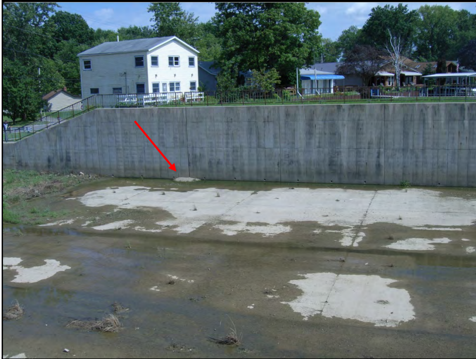
BUCKEYE LAKE 25 AUGUST 2014 Photo 021 – View from west side of Sellers Point spillway. Note the large amount of eroded material deposited along the base of east training wall.
