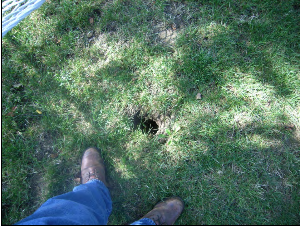
BUCKEYE LAKE 25 AUGUST 2014 Photo 037 – Several depressions approximately 3.6 feet deep were noted near the center of the embankment crest between Stations 129+16 to 139+70.
