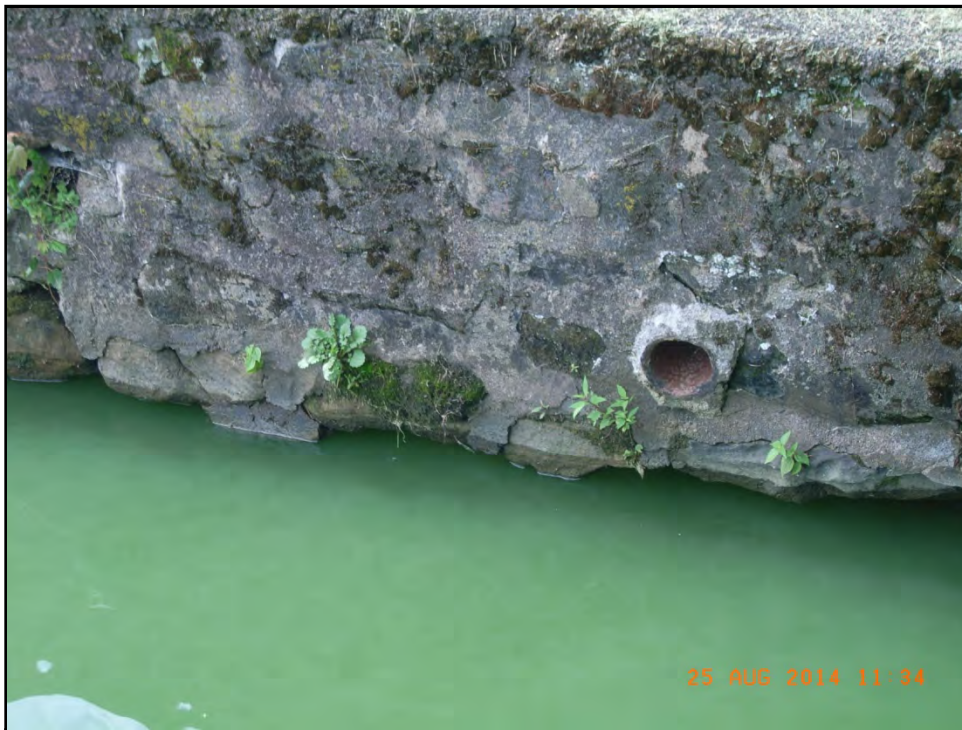
BUCKEYE LAKE 25 AUGUST 2014 Photo 006 – Drainage pipes penetrate through the masonry wall along the west embankment.
