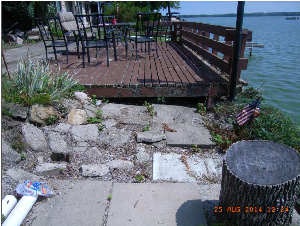
BUCKEYE LAKE 25 AUGUST 2014 Photo 012 – Wood decks and patio structures inhibit monitoring the crest of the dam for signs of distress. Additionally they preclude grass growth which provides erosion protection of this earthen dam.
