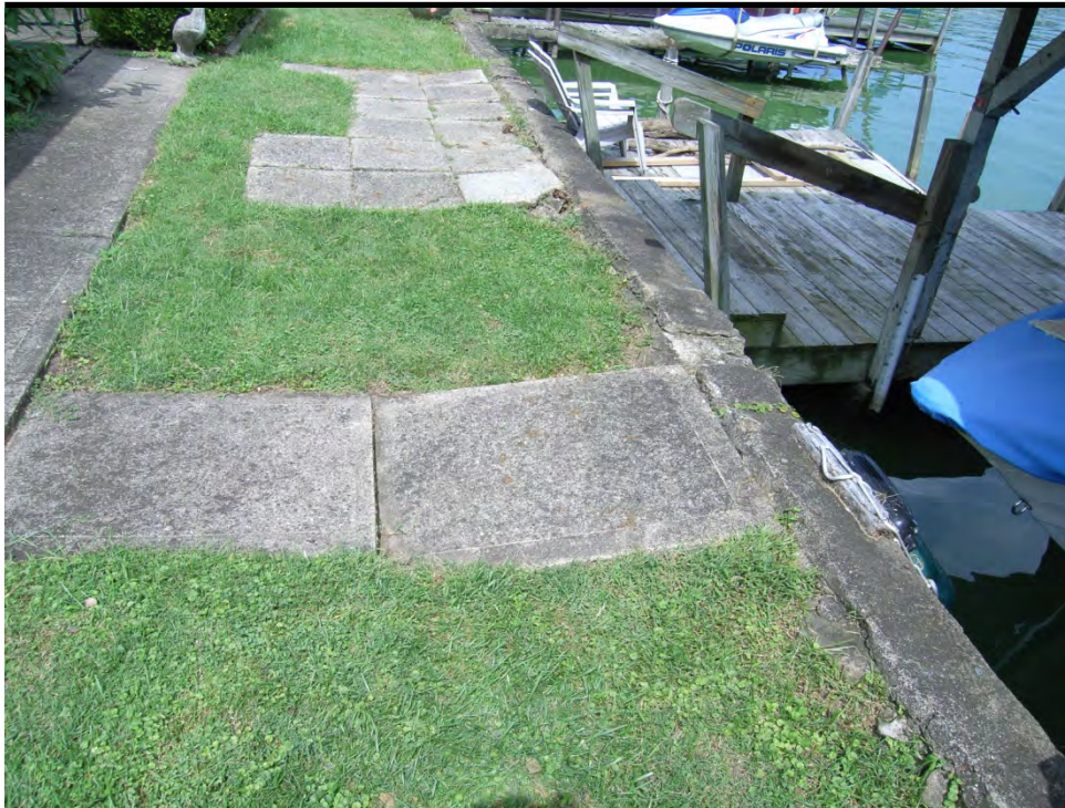
BUCKEYE LAKE 25 AUGUST 2014 Photo 005 – Typical settlement feature observed behind the masonry wall along the west embankment.
