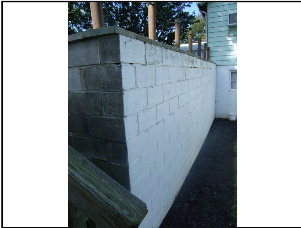
BUCKEYE LAKE 25 AUGUST 2014 Photo 036 – Concrete masonry unit wall with numerous cracks.
