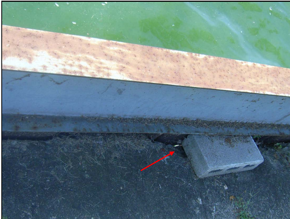
BUCKEYE LAKE 25 AUGUST 2014 Photo 046 – Thinning and loss of sheetpile wall. Holes were observed through the wall. The wall beneath the water surface was not observed during the August inspection.
