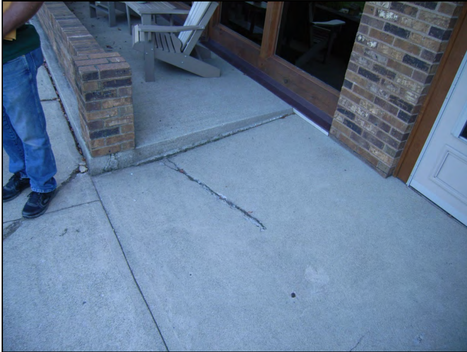
BUCKEYE LAKE 25 AUGUST 2014 Photo 023 – Cracks in sidewalks and porches along the crest of the dam and adjacent to houses which formed as a result of embankment displacement along northern dam reach.
