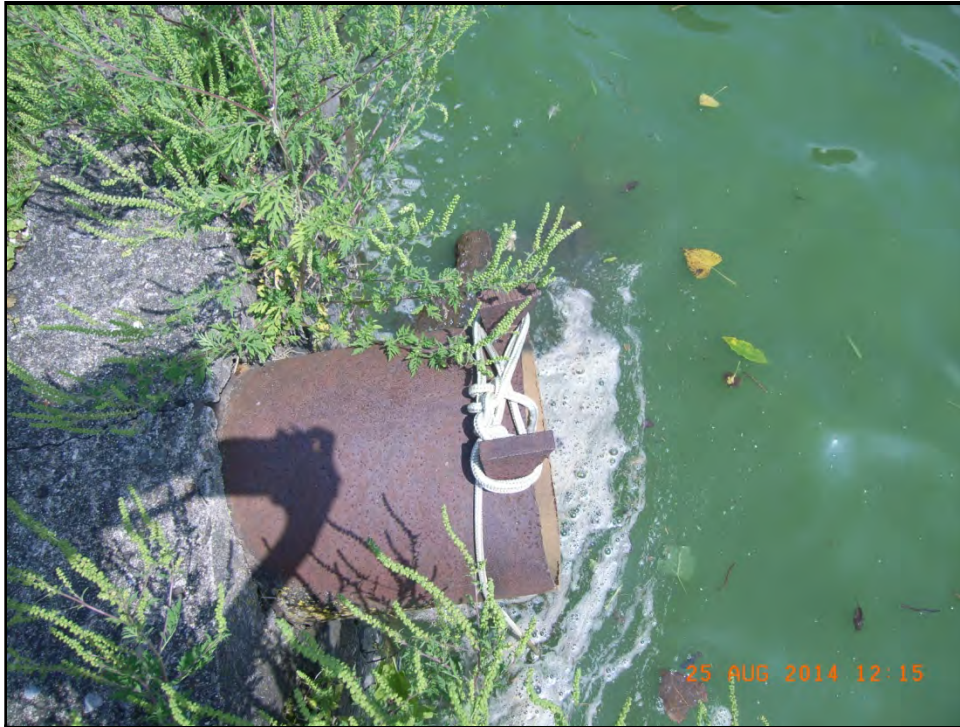
BUCKEYE LAKE 25 AUGUST 2014 Photo 011 – Flap gate on a drainpipe connecting the pool to a downstream lagoon is missing.
