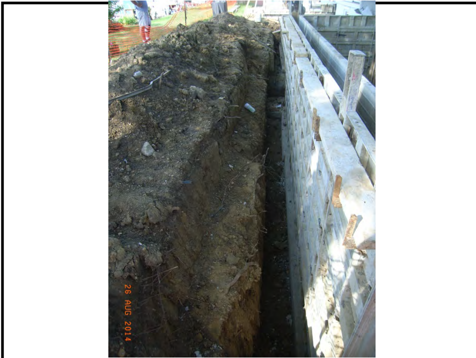
BUCKEYE LAKE 25 AUGUST 2014 Photo 044 – Unsupported excavation into embankment.
