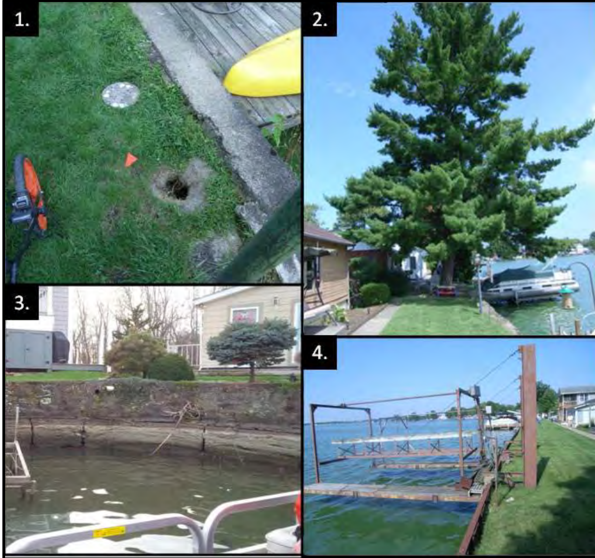
Figure 2. Typical Distress Observations 1) One of many depressions behind masonry wall 2) Tree with root system spanning the entire embankment crest 3) Numerous cracks within base of, and pipe/utility penetrations through, masonry wall observed during winter pool drawdown 4) Dock structures cantilevering from the dam put stress on the sheetpiling for which it was not designed
