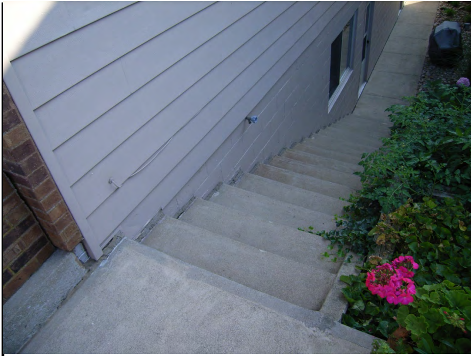
BUCKEYE LAKE 25 AUGUST 2014 Photo 024 – Another photograph of same structure in Photo 023. Note that the sidewalk is misaligned with structure indicating embankment displacement.
