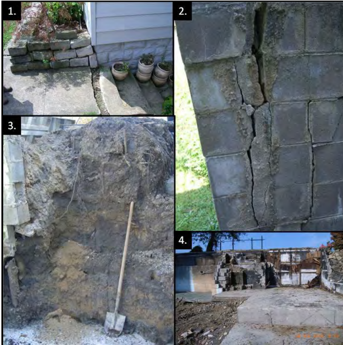
Figure 1. Typical Embankment Distress Observations 1) Differential settlement of structure built into crest/embankment longitudinal cracking 2) Failing masonry unit wall supporting landside embankment materials 3) Unsupported excavation into downstream face of embankment which could cause weakening of embankment soils and embankment failure 4) Several rows of masonry unit walls were noted in old house foundations likely indicating seepage related displacement
