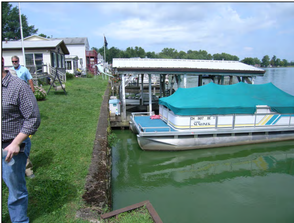
BUCKEYE LAKE 25 AUGUST 2014 Photo 002 – Masonry wall alignment as seen from west abutment.
