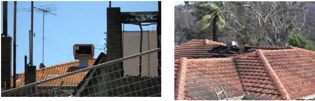
Figure 14: Two further homes with evaporative air conditioners and fire affected
