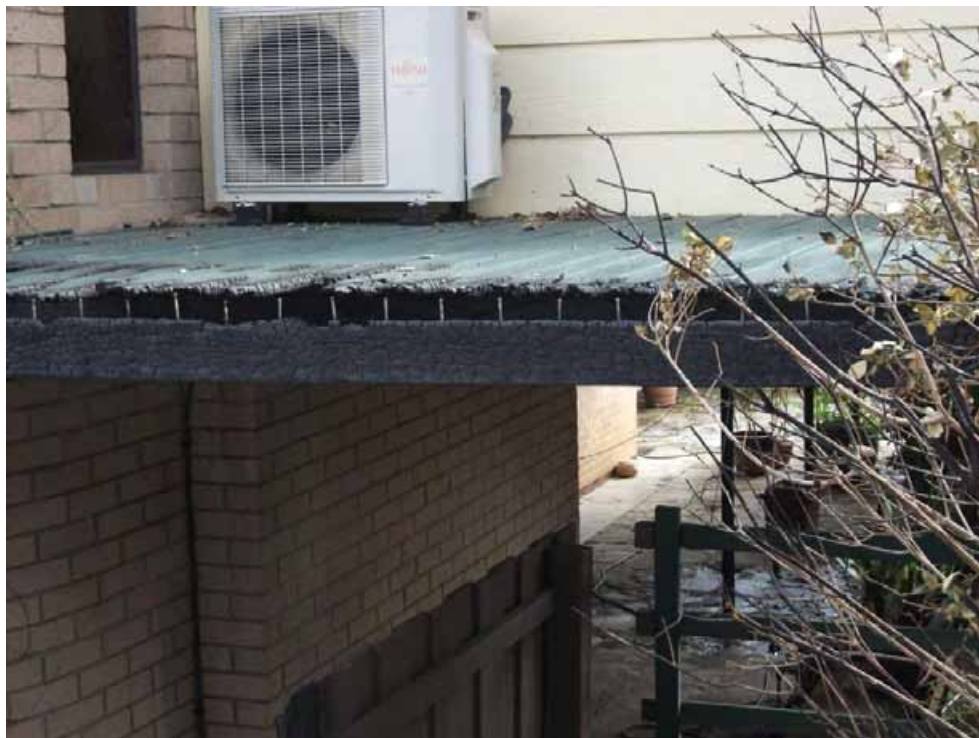
Figure 31: House damage following the tall plants igniting and putting direct flame contact onto the house
