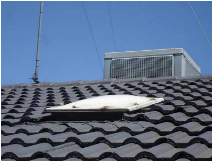
Figure 25: Ember caused damage to a sky light
