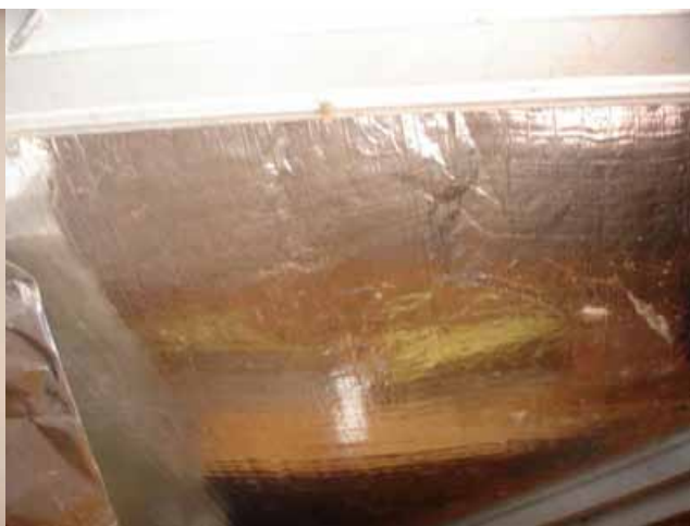
Figure 35: Shows the sarking through the broken cement sheet
