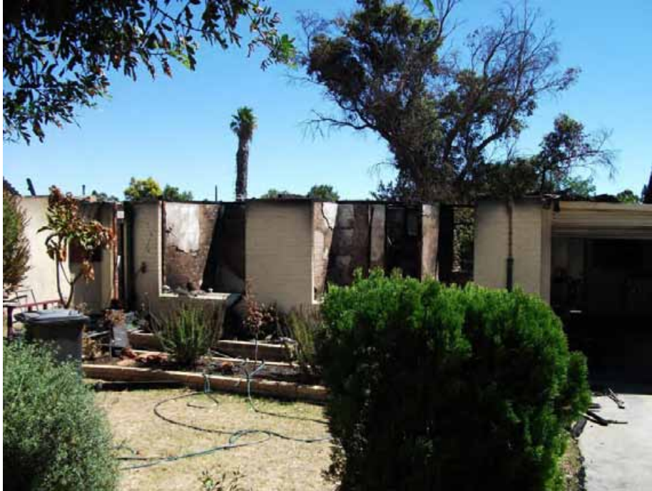
Figure 12: A home destroyed by ember attack. This home was 421 metres from the fire. This home also had a roof mounted evaporative air conditioner
