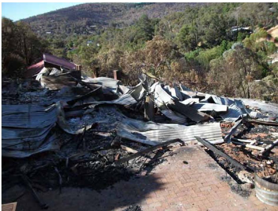
Figure 20: A cedar timber home destroyed following an ember attack
