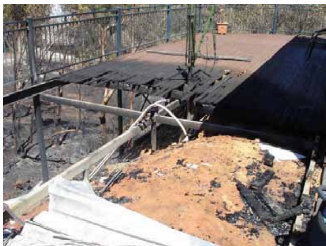
Figure 32: Shows the deck damage
