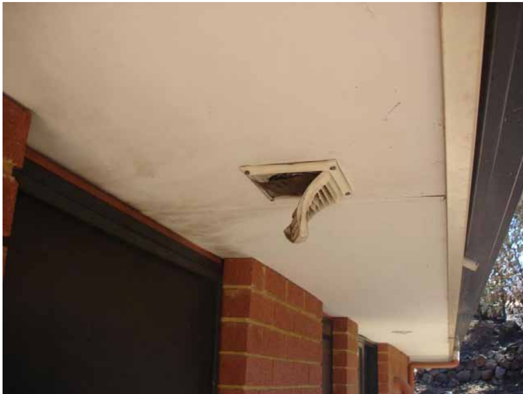
Photograph 37: The melted air vent and smoke staining on the eaves.
