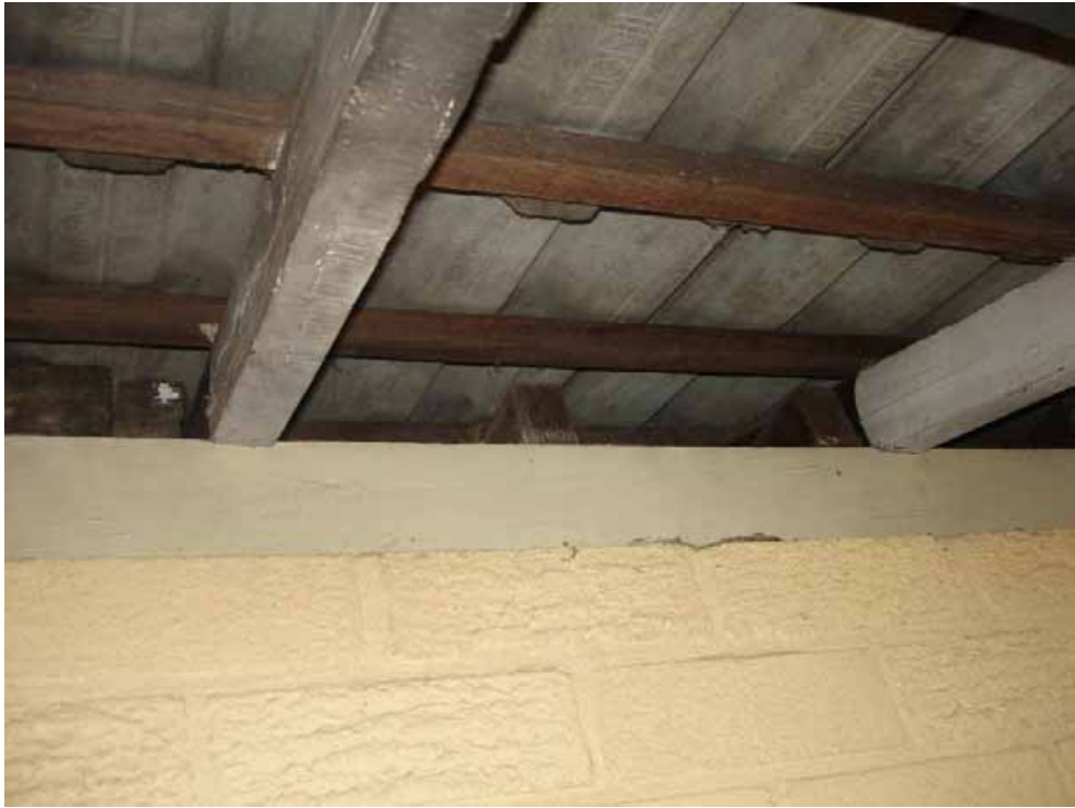
Figure 16 : This home was constructed without ember proofing. This house was on Martin Road and was subject to ember attack.
