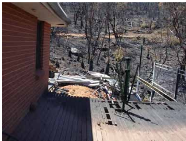
Figure 33: Shows the deck damage and BPZ vegetation structure
