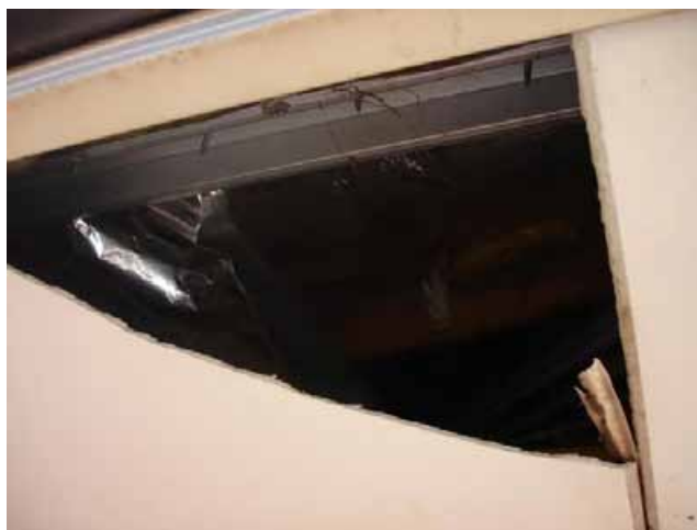
Figure 34: Shows the broken cement sheet
