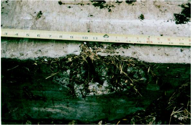
Anchor bolt pulled from side of slab foundation
