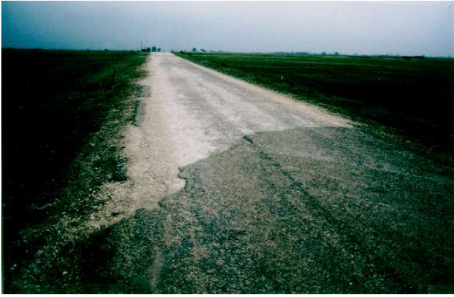
Asphalt road pavement removed by Jarrell tornado
