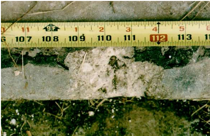
Nail pulled from side of slab foundation
