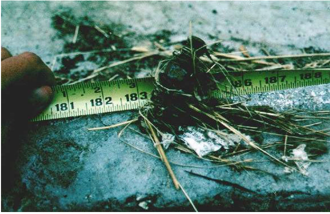
Bent anchor bolt which secured bottom plate to slab -- grass around bolt shows wind direction
