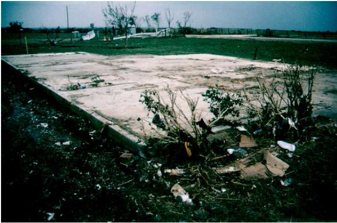
Home swept from concrete slab foundation
