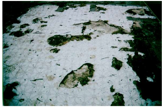
Gouges in vinyl flooring from flying debris
