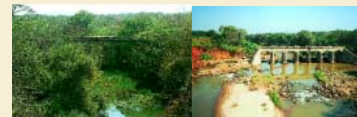
Photographs taken from the same road bridge across the Latonyanda River before the 2000 floods and after (April 2001).
