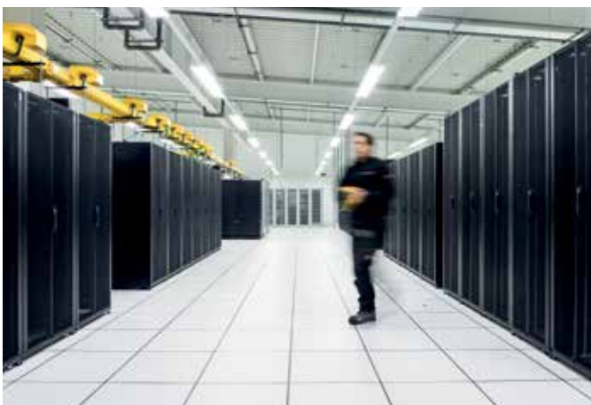
Data centre floor
