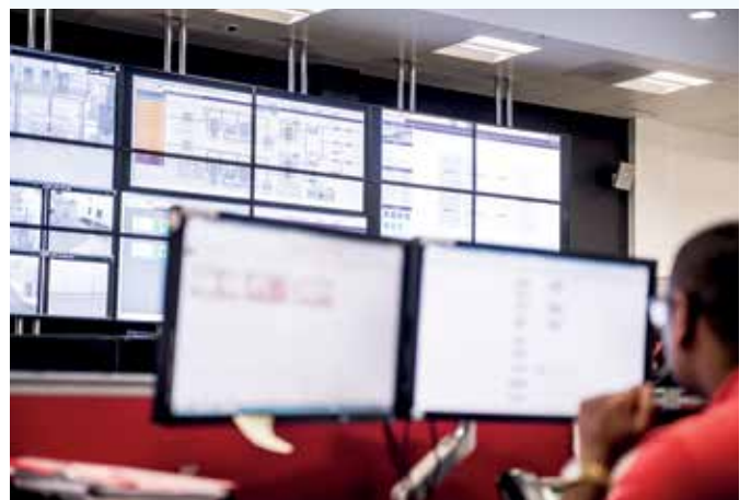
Network operations centre
