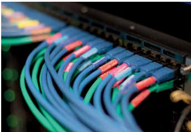
A patching panel where customers interconnect their networks
