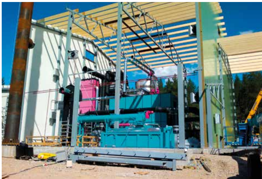
KWK-Anlage von Polytechnik in Posio in Lapland CHP plant from Polytechnik in Posio in Lapland
