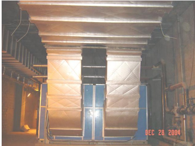
Platform Air Handling Unit
