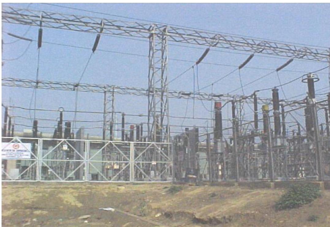
Typical High Voltage Receiving Sub-station
